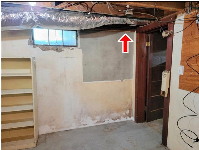
1.9 Item 1(Picture) Rim Joist Damage (Basement Front Wall)
