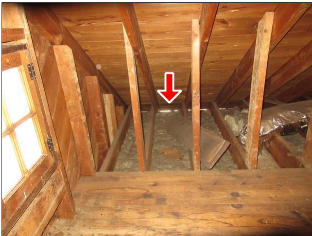
1.7 Item 1(Picture) Gap (Around Perimeter)
