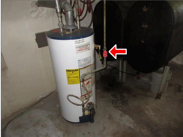
3.8 Item 1(Picture) Gas Water Heater Valve
