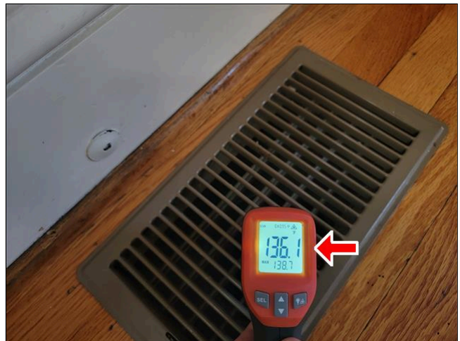
2.1.B Item 2(Picture) 136.1 Degrees (Heat Stage 2 "Aux")
