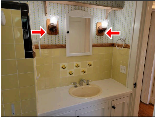
4.5 Item 1(Picture) Upstairs Bathroom Outlets
