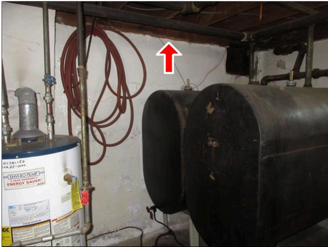
1.9 Item 3(Picture) Sill and Rim Joist Damage (Left Wall)
