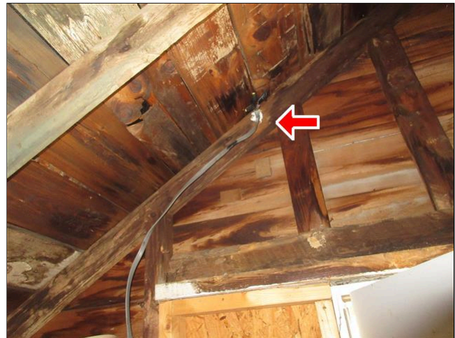
9.6 Item 2(Picture) Disconnected Electrical
