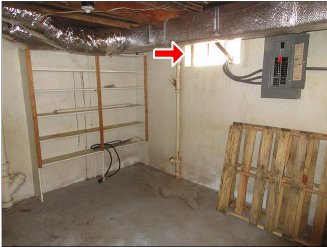
1.6 Item 7(Picture) Cracked Glass (Basement)
