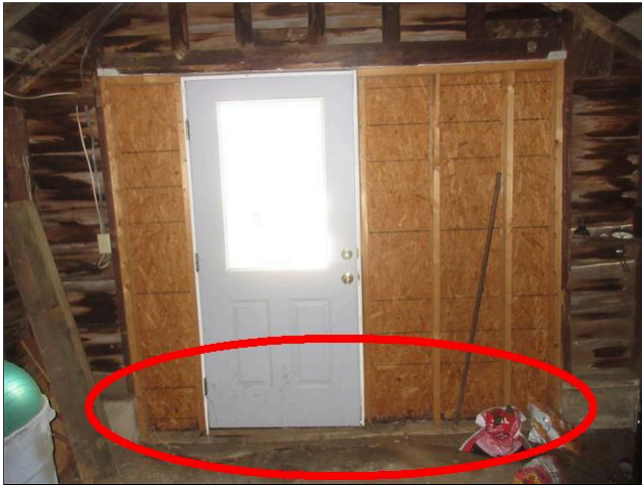
9.6 Item 3(Picture) Interior Staining
