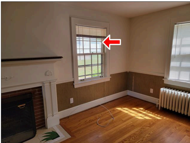
1.6 Item 5(Picture) Cracked Glass (Living Room)
