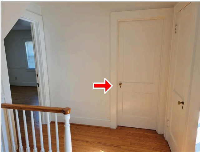
1.5 Item 1(Picture) Upstairs Left Rear Room (Not Latching/Missing Strike Plate)
