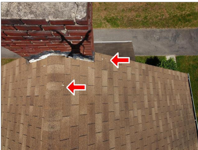
8.0 Item 3(Picture) Exposed Nail Heads (Around Chimney Flashing and Ridge Shingle
