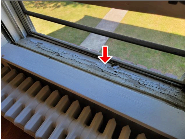
1.8 Item 1(Picture) Peeling Paint Chips (Most Window Sills)
