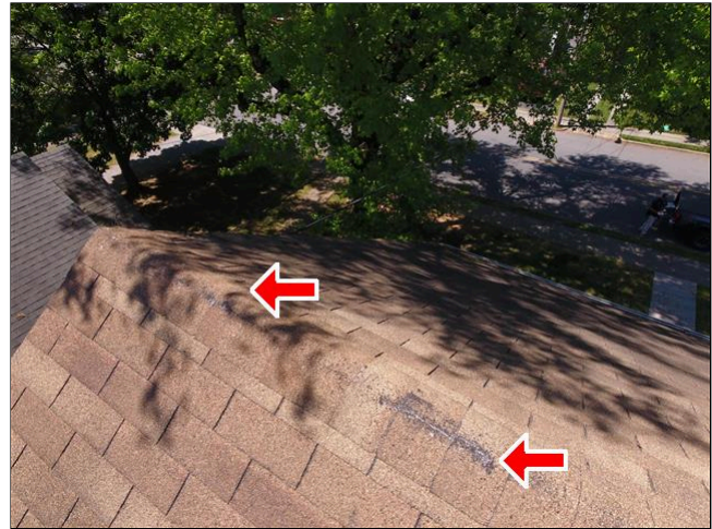
8.0 Item 6(Picture) Ridge Shingle Damage
