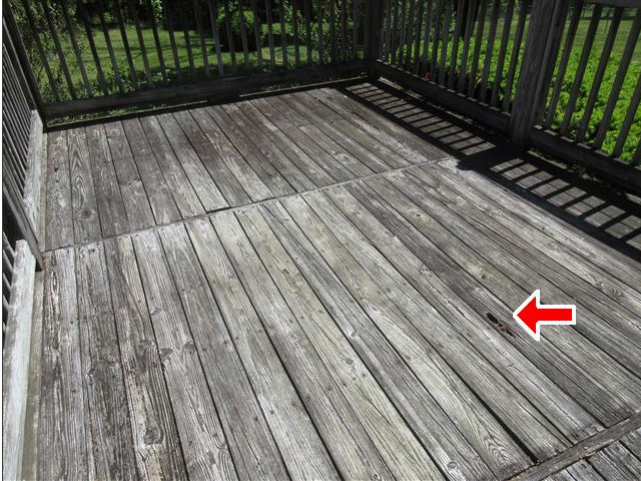
9.3 Item 1(Picture) Deterioration (Decking)
