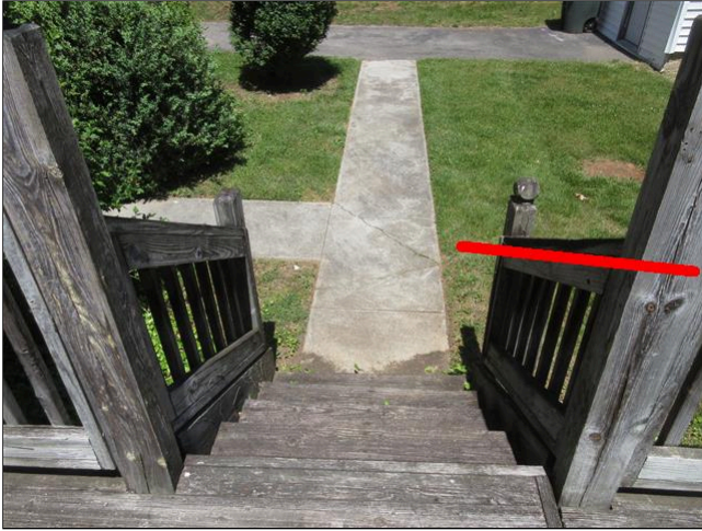
1.3 Item 3(Picture) Exterior Deck (No Handrail)
