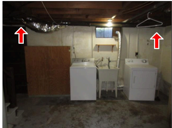
1.9 Item 2(Picture) Rim Joist Damage (Basement Front Wall)
