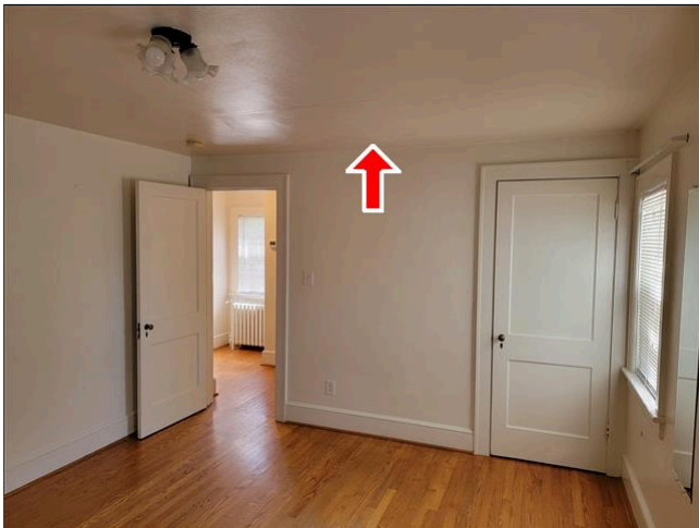
1.0 Item 1(Picture) Upstairs Right Side Bedroom (Staining and Repairs - Air Handler Above)
