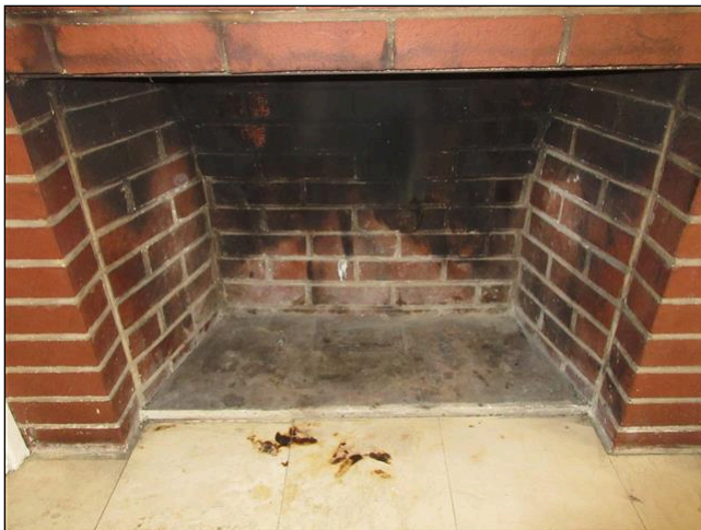
2.6.B Item 1(Picture) Cracking and Open Joints (Living Room Fireplace)
