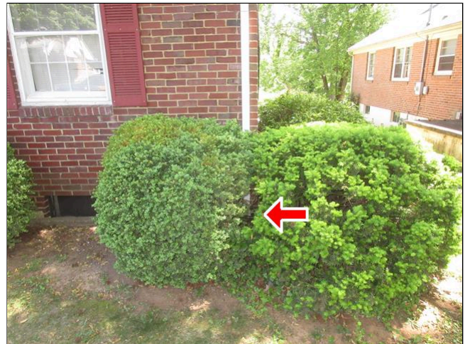
8.3 Item 2(Picture) Front Right Discharge
