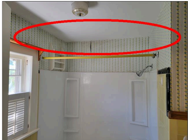
1.0 Item 2(Picture) Mildew (Upstairs Bathroom)
