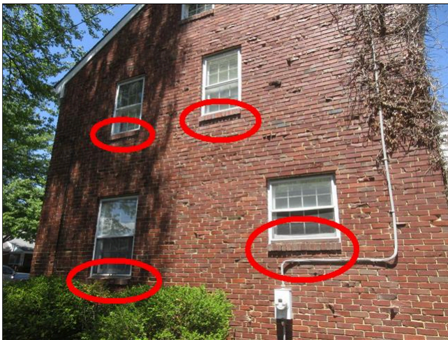
9.0 Item 7(Picture) Open Joints (Right Side)
