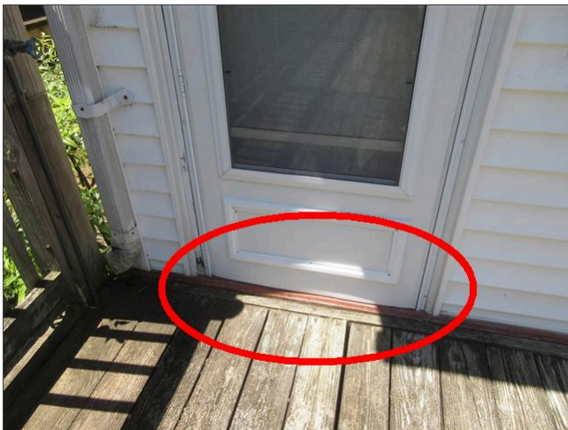
9.0 Item 3(Picture) Openings and Deterioration (Rear)
