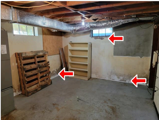
1.9 Item 4(Picture) Staining, Spalling and Mildew/Organic Growth (Multiple Areas)
