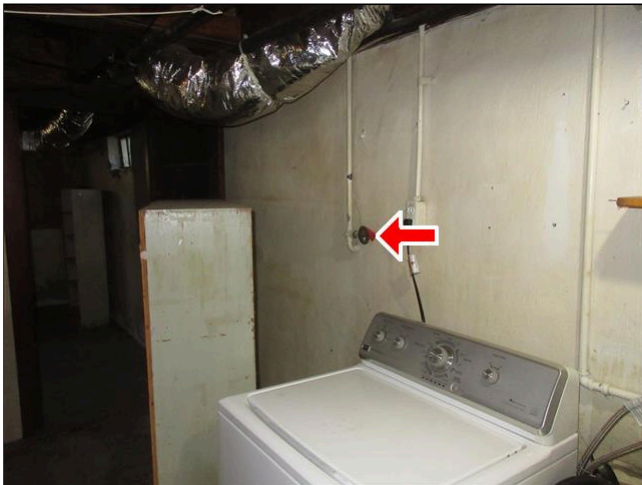
3.6 Item 1(Picture) Main Valve
