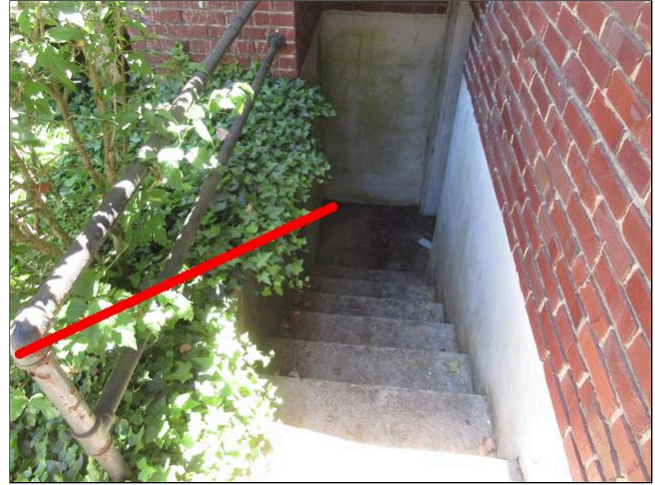
1.3 Item 4(Picture) Exterior Basement Stairwell (No Handrail and Horizontal Balusters)
