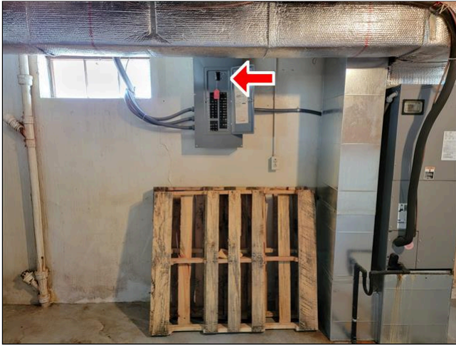
4.10 Item 1(Picture) Main Breaker
