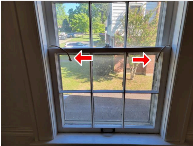
1.6 Item 1(Picture) Broken Balance Cords (Multiple Windows)
