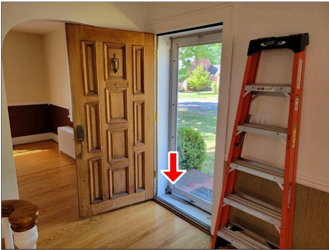
9.1 Item 1(Picture) Damaged Closer (Front Storm Door)
