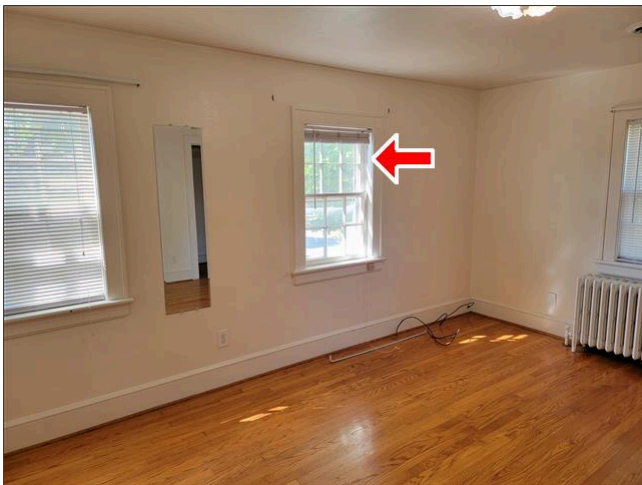
1.6 Item 3(Picture) Cracked Glass (Upstairs Right Bedroom)
