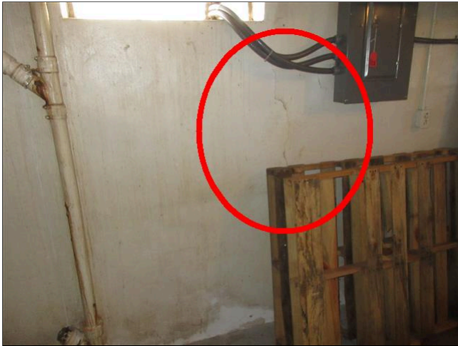
1.9 Item 6(Picture) Spalling/Cracking
