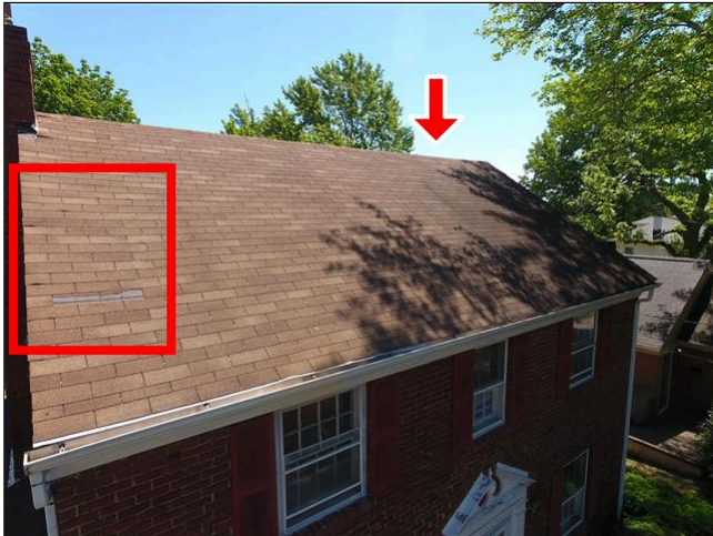
8.0 Item 1(Picture) Wind Lift Damage, Exposed Nail Heads, Nail Pops, and Shingle Damage
