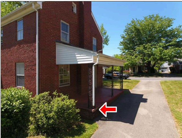
8.3 Item 1(Picture) Left Discharge (Mortar Deterioration)
