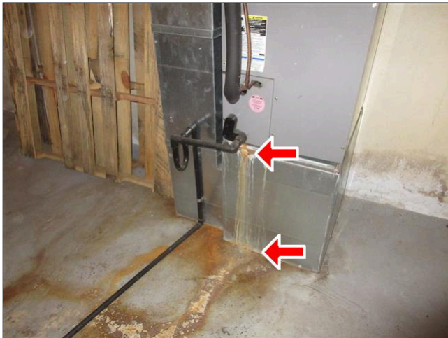
2.2.B Item 1(Picture) Staining
