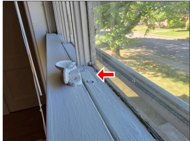
1.6 Item 2(Picture) Missing Lock Hardware (Multiple Windows Including Ground Access)
