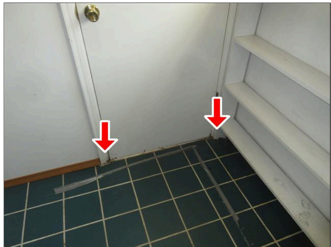
9.0 Item 4(Picture) Interior Staining (Rear Entrance)
