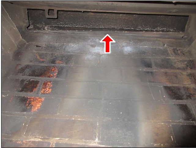
2.5.B Item 1(Picture) No Damper (Living Room)
