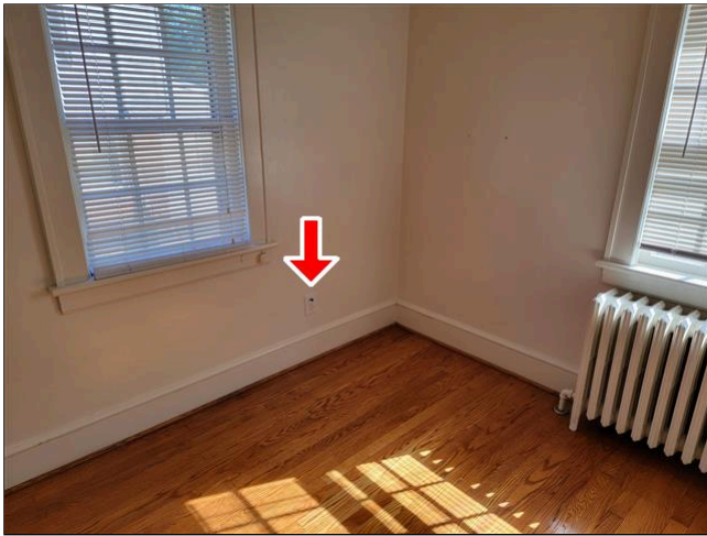
4.4 Item 1(Picture) Broken Outlet (Upstairs Left Rear Room)
