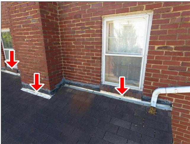
8.0 Item 7(Picture) Exposed Nail Heads (Sidewall Flashing)
