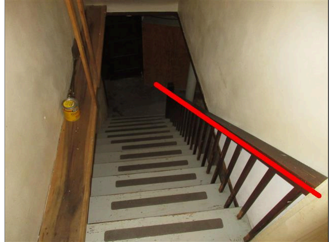
1.3 Item 2(Picture) Basement Stairwell (No Handrail)
