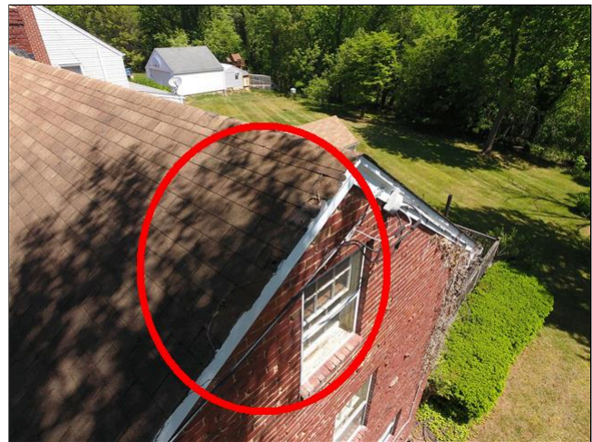
8.0 Item 8(Picture) Damaged Shingles and Exposed Roof Sheathing (Front Right)
