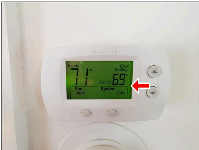
2.10.B Item 3(Picture) Thermostat Setting
