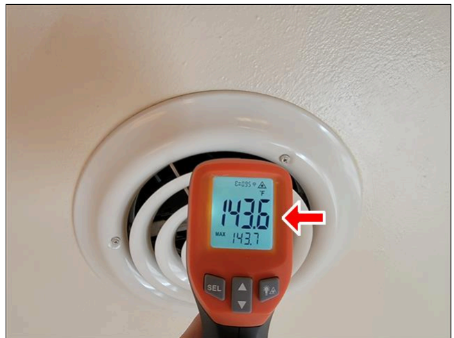
2.1.A Item 2(Picture) 143.6 Degrees (Heat Stage 2 "Aux")
