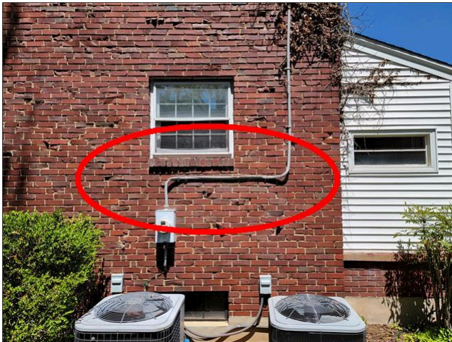
4.1 Item 1(Picture) Deteriorated Sheathing
