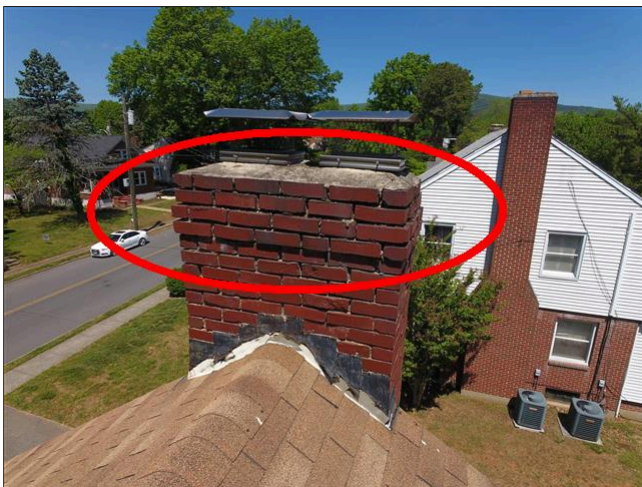
6.6 Item 1(Picture) Mortar Joint Deterioration
