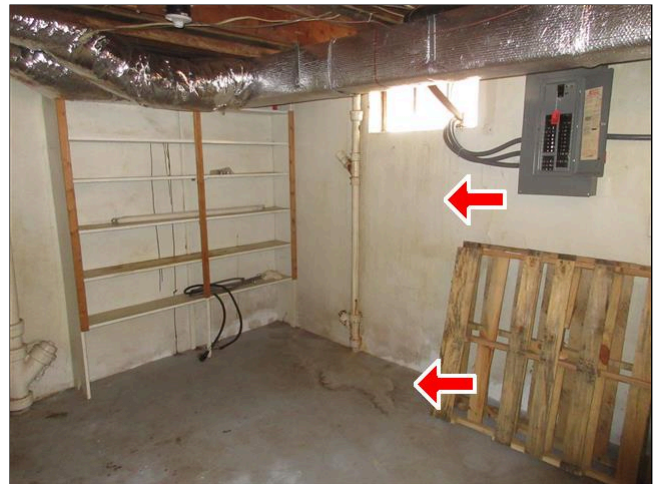
1.9 Item 5(Picture) Staining and Spalling
