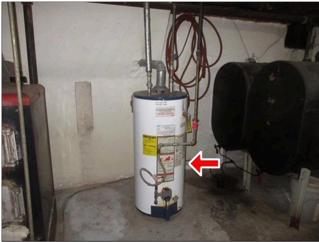
3.5 Item 1(Picture) Water Heater
