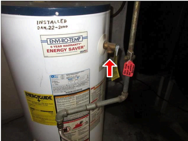
3.3 Item 1(Picture) No Discharge Tube
