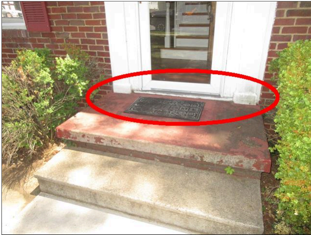
9.0 Item 5(Picture) Open Joints (Around Front Entrance)
