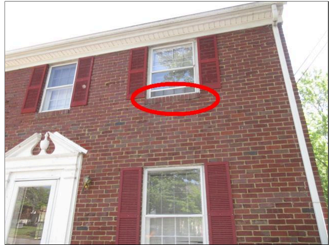
9.0 Item 6(Picture) Open Mortar Joints (Front Right)
