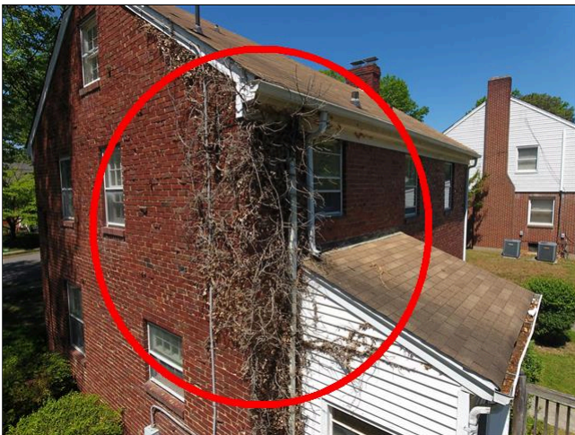
9.4 Item 1(Picture) Dead Overgrowth (Right Rear Corner)
