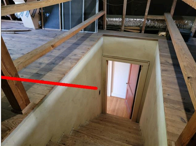
1.3 Item 1(Picture) Attic Stairwell (No Handrail and Horizontal Balusters)
