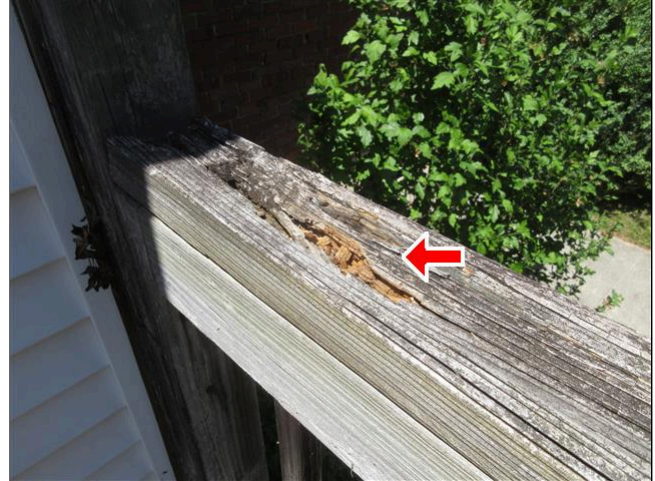
9.3 Item 2(Picture) Deterioration (Top Rail)
