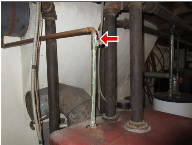
3.2 Item 1(Picture) Active Leak
