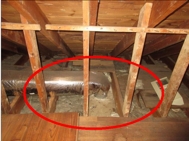
7.0 Item 1(Picture) Little Insulation and Missing Insulation
