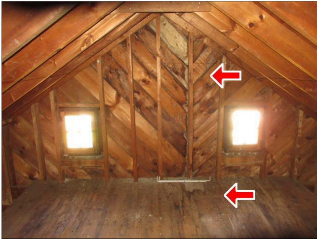
8.0 Item 5(Picture) Staining (Chimney Side)
