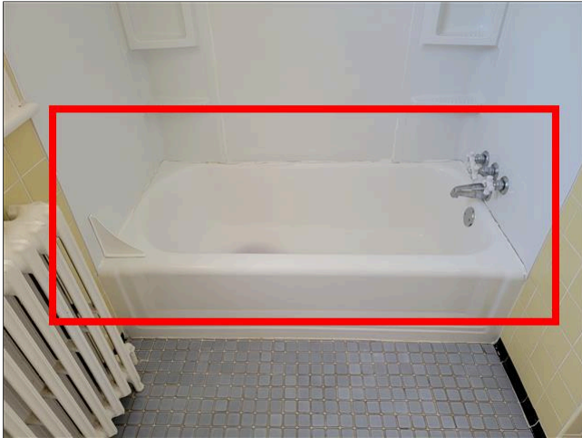
1.1 Item 2(Picture) Open Joints
