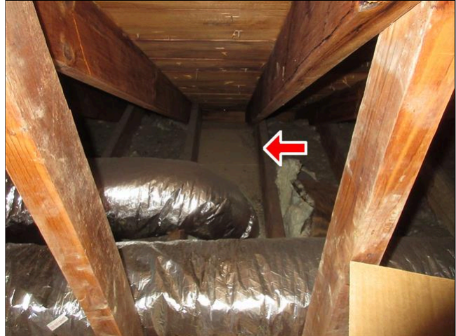
7.0 Item 2(Picture) Little Insulation and Missing Insulation
