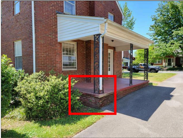
9.0 Item 1(Picture) Mortar Deterioration and Loose Bricks (Left Side)
