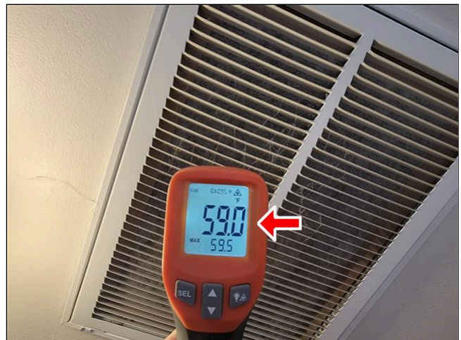
2.10.A Item 2(Picture) 59 Degrees (Return Air)
