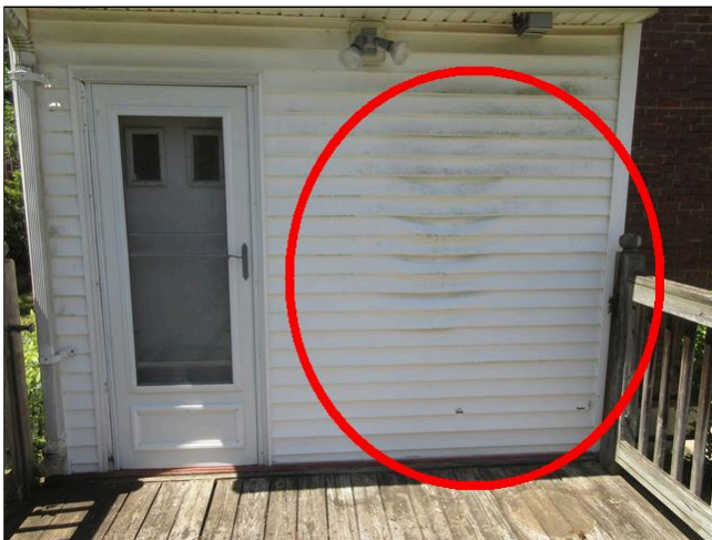
9.0 Item 9(Picture) Siding Disruptions and Holes (Rear)
