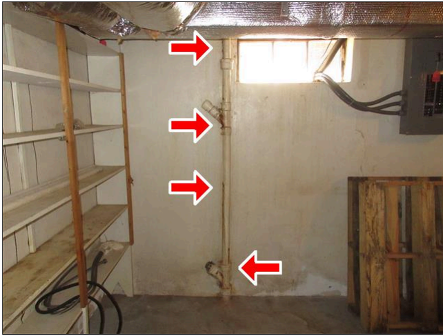
3.0 Item 1(Picture) Waste Line Deterioration and Staining
