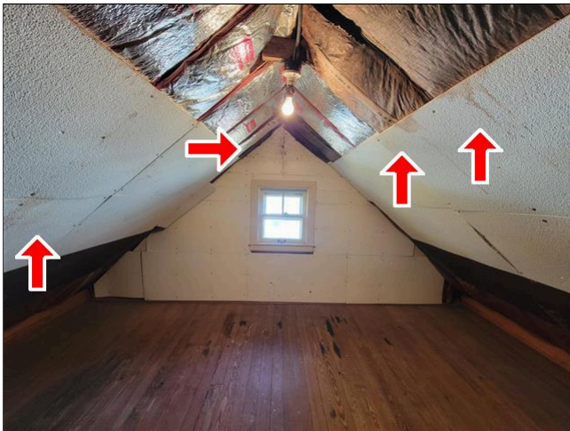
1.0 Item 1(Picture) Staining and Potential Organic Growth (Left Access)
