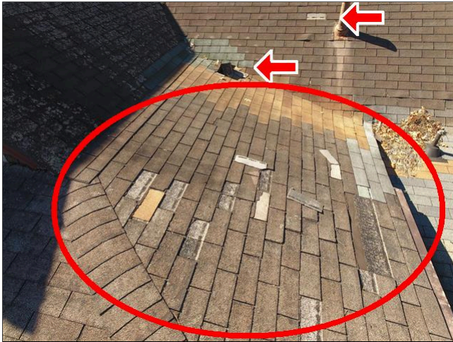
8.0 Item 5(Picture) Missing Shingles and Exposed Nail Heads
