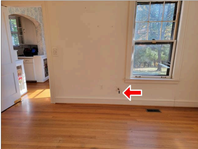
4.4 Item 1(Picture) Inactive 220 Outlet (Dining Room)
