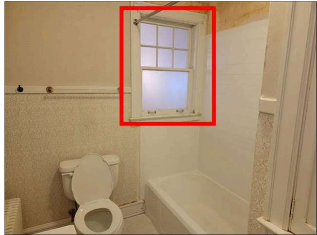
1.6 Item 6(Picture) No Safety Glass (Main Bathroom Shower)
