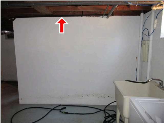
1.9 Item 10(Picture) Location (Near Washing Machine)
