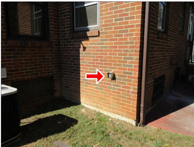
4.5 Item 4(Picture) Grounded (Exterior Outlet)
