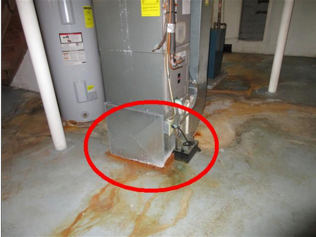
2.2 Item 1(Picture) Corrosion
