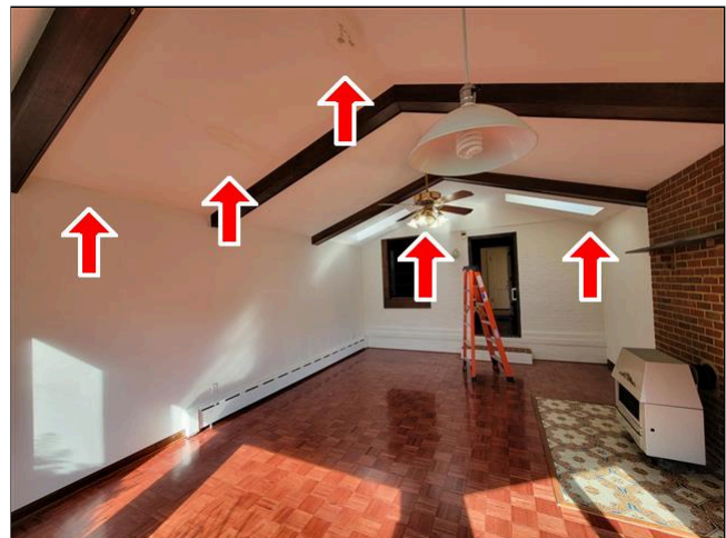
1.0 Item 4(Picture) Staining (Right Side Den)
