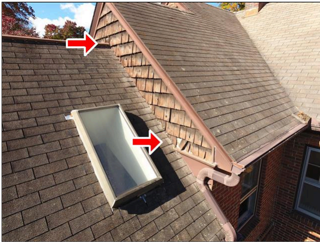
9.0 Item 1(Picture) Damaged Wood Siding and Openings
