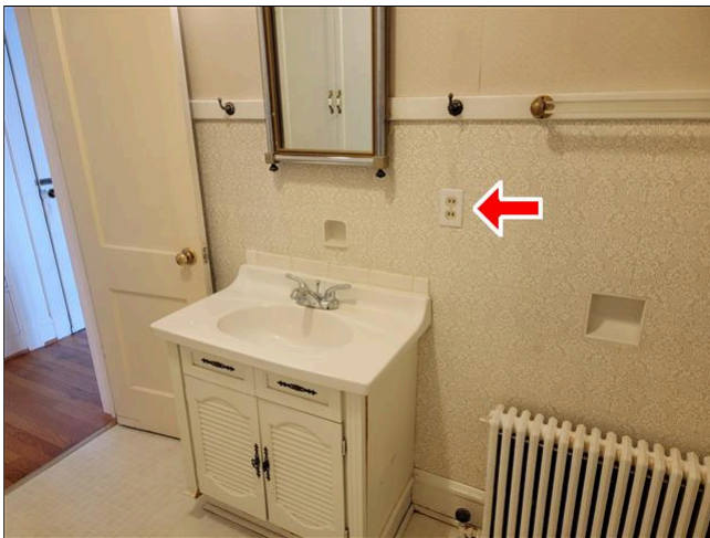
4.5 Item 1(Picture) Ungrounded (Main Bathroom)
