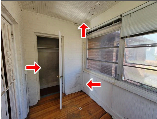
1.0 Item 5(Picture) Staining, Moisture, and Organic Growth (Rear Mud Room)
