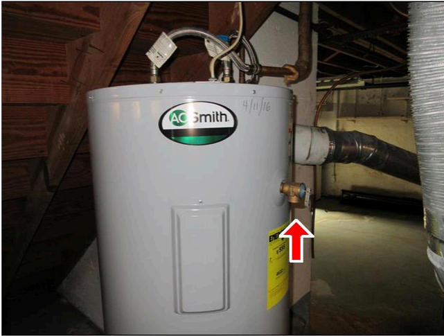
3.3 Item 1(Picture) No Discharge Tube
