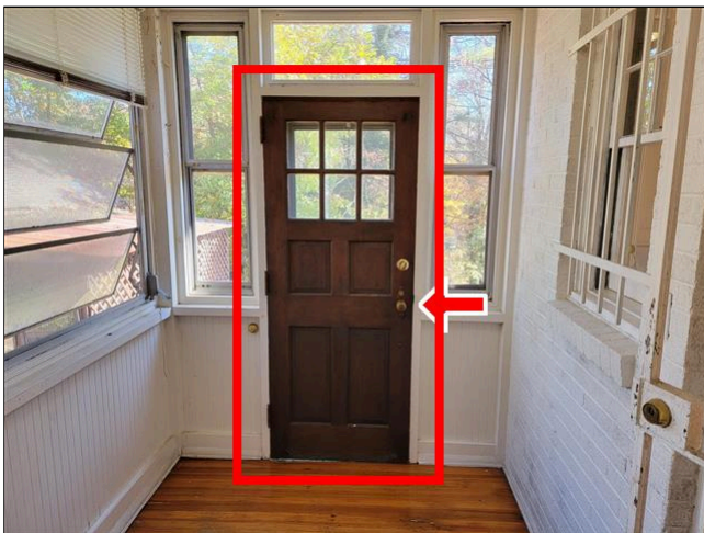
9.1 Item 1(Picture) No Weather Stripping and Faulty Door Knob (Rear)
