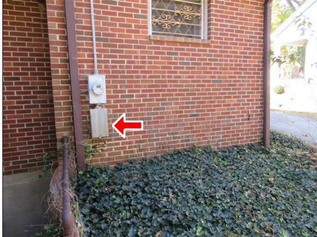
4.10 Item 1(Picture) Exterior Disconnect Panel
