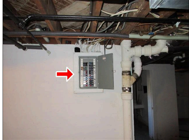
4.10 Item 2(Picture) Main Interior Panel/ Breakers
