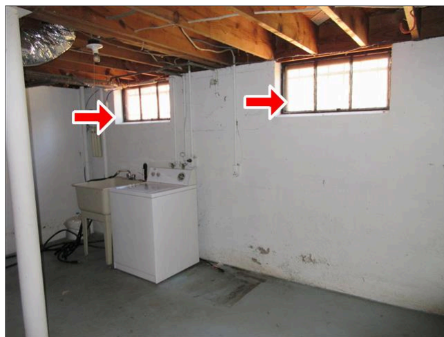
1.6 Item 2(Picture) Broken/ Cracked Glass (Basement)
