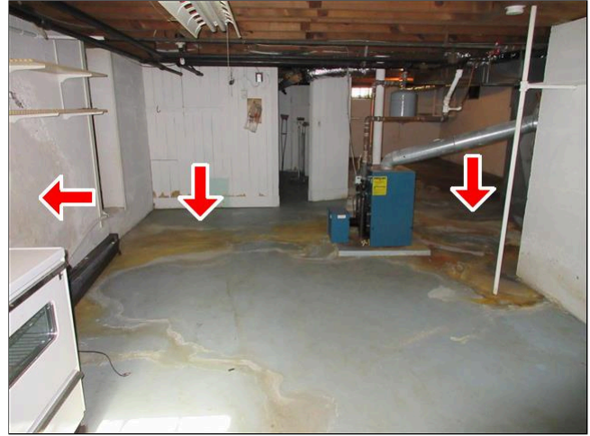
1.9 Item 4(Picture) Staining
