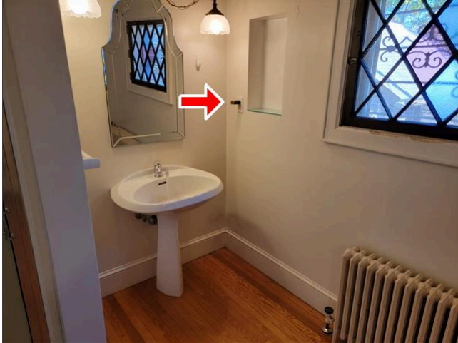
4.6 Item 1(Picture) Faulty GFCI Outlet (Primary Bathroom)
