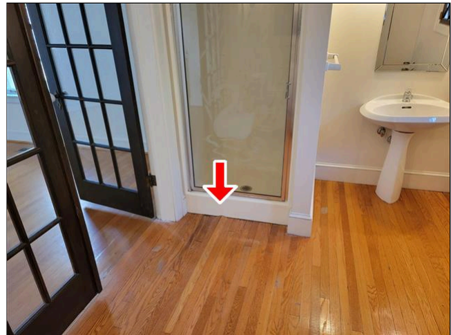
1.2 Item 2(Picture) Disruptions (Primary Bathroom)
