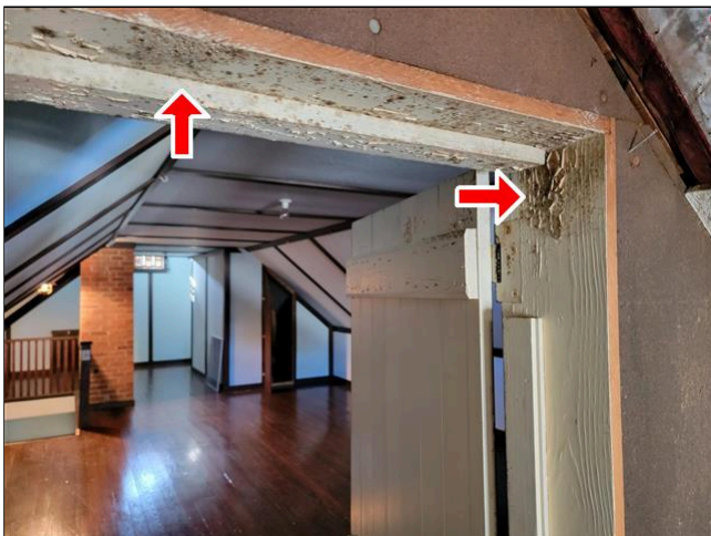
1.0 Item 3(Picture) Additional View of Potential Growth and Peeling Paint
