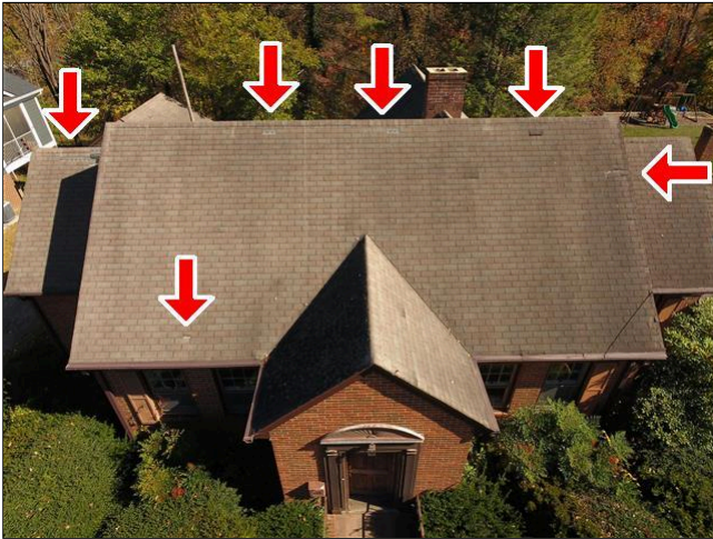
8.0 Item 1(Picture) Wind Lift, Missing Tabs, and Nail Pops
