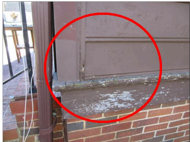
9.0 Item 4(Picture) Deterioration and Peeling Paint
