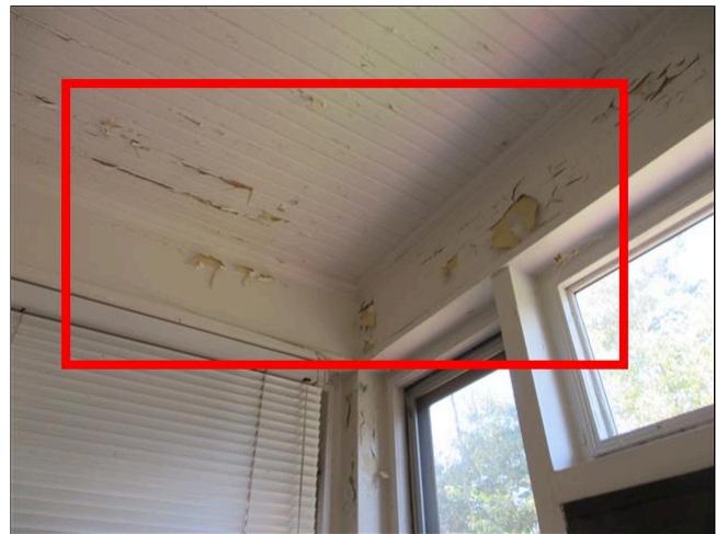
1.8 Item 2(Picture) Paint Chips (Multiple Locations)
