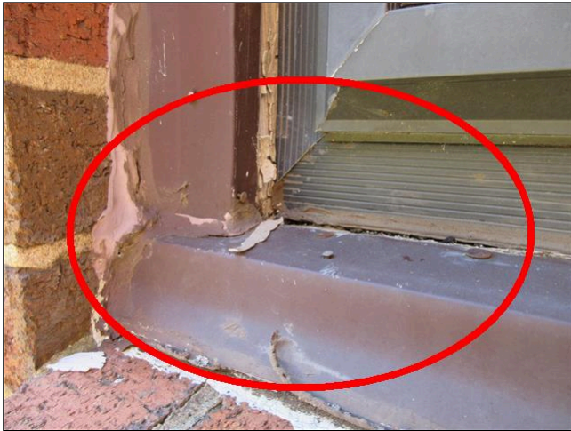
9.0 Item 5(Picture) Openings and Failing Sealant (Around Windows)
