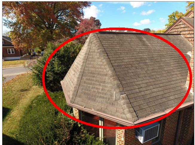
8.0 Item 4(Picture) Substantial Granular Loss, and Damaged Shingles
