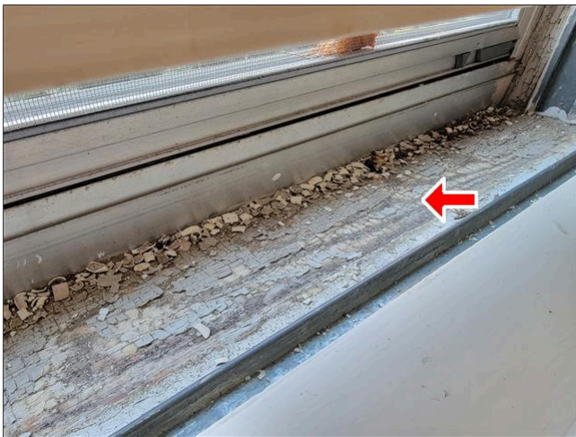
1.8 Item 1(Picture) Paint Chips
