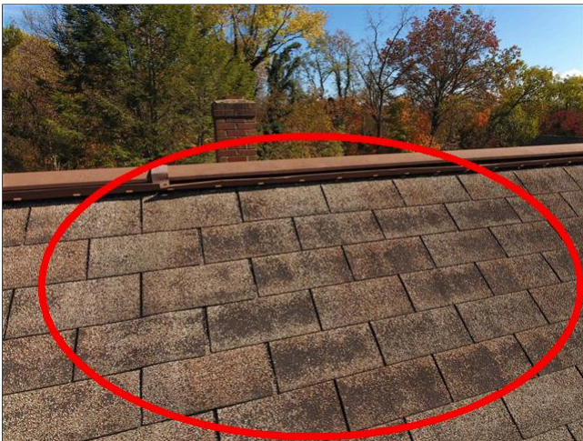
8.0 Item 3(Picture) Substantial Granular Loss
