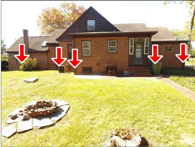
8.3 Item 1(Picture) Discharge (Multiple Locations Around the Exterior Front and Rear)
