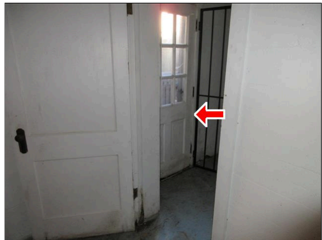
9.1 Item 2(Picture) Not Closing (Basement)
