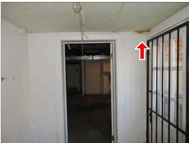
1.0 Item 7(Picture) Staining and Organic Growth (Above Basement Entrance)
