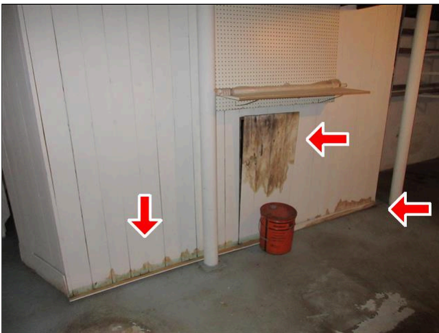
1.9 Item 7(Picture) Staining and Organic Growth
