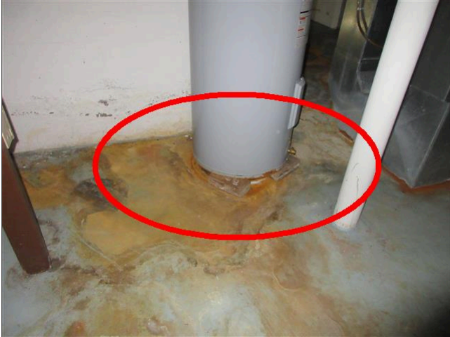
3.3 Item 3(Picture) Corrosion
