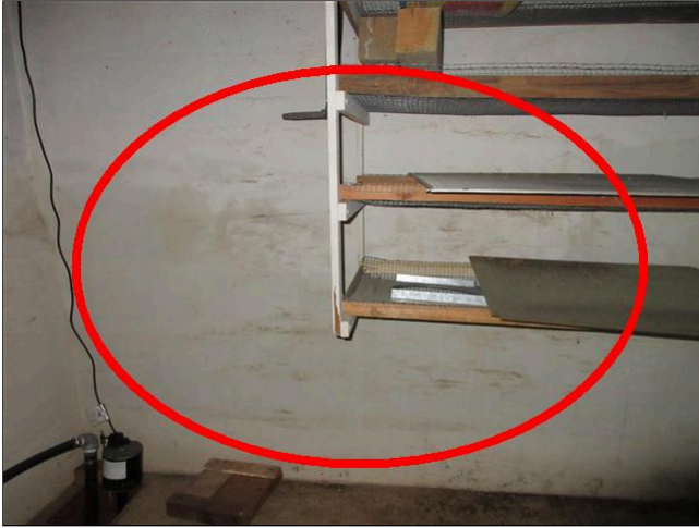
1.9 Item 3(Picture) Staining, Efflorescence, and Organic Growth (Basement Front Storage Area)
