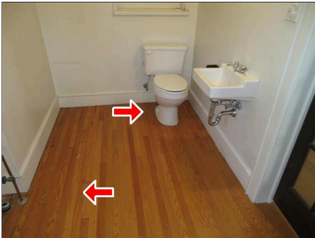
1.2 Item 1(Picture) Loose Flooring and Slope (Primary Bathroom)
