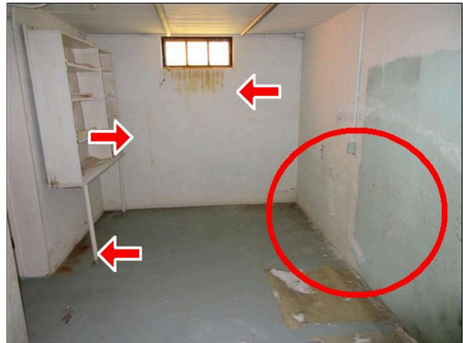
1.9 Item 2(Picture) Staining, Efflorescence (Basement Storage Cellar)
