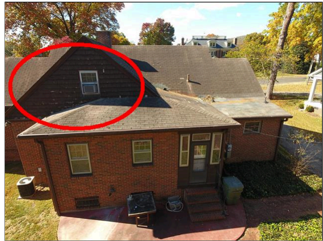
9.0 Item 2(Picture) Damaged Wood Siding and Openings
