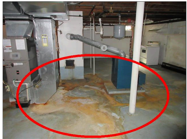
1.9 Item 6(Picture) Staining
