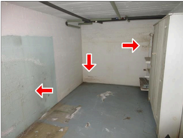
1.9 Item 1(Picture) Staining, Efflorescence, and Organic Growth (Basement Storage Cellar)
