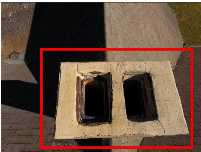
6.6 Item 1(Picture) Cracking (Middle Chimney)
