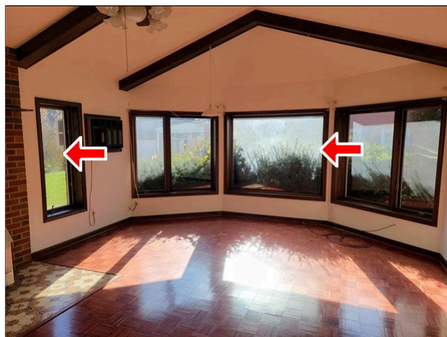
1.6 Item 4(Picture) Failed Seals (Right Side Den)
