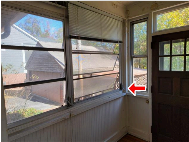
1.6 Item 5(Picture) Faulty Crank Assembly
