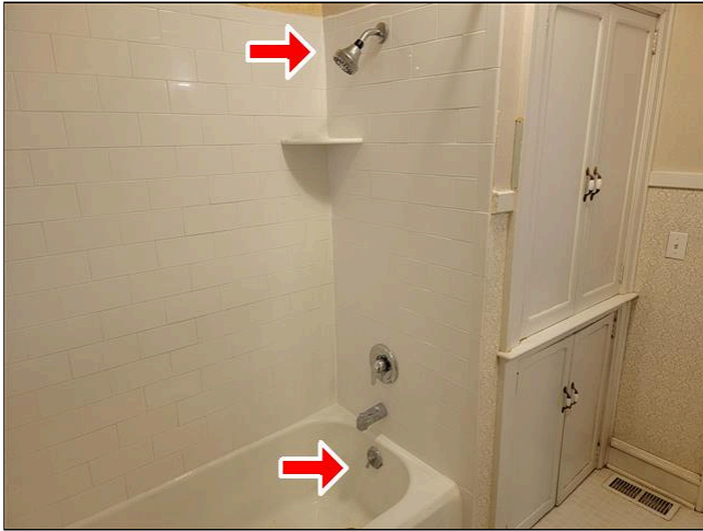
3.2 Item 1(Picture) Loose Shower Head Mount and Faulty Stopper (Main Bathroom)
