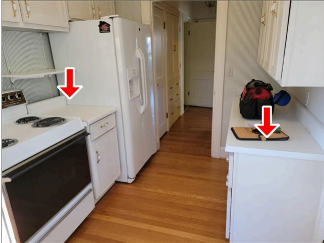
1.4 Item 1(Picture) Loose Countertops
