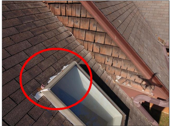
8.0 Item 2(Picture) Damaged Shingles (Around Skylights)
