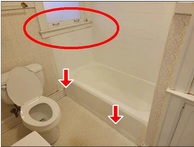
1.1 Item 1(Picture) Open Joints (Around Main Bathroom Shower and Window)
