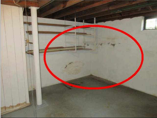
1.9 Item 9(Picture) Staining and Efflorescence
