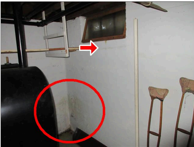
1.9 Item 5(Picture) Staining and Efflorescence
