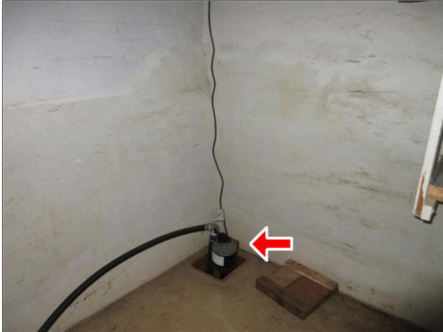
3.5 Item 1(Picture) Sump Pump
