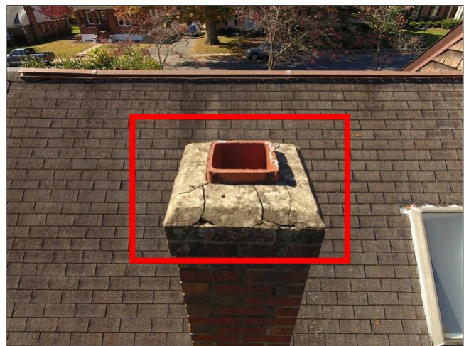
6.6 Item 2(Picture) Cracking (Right Rear Chimney)
