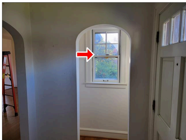
1.6 Item 1(Picture) Broken Glass (Right of the front entrance)
