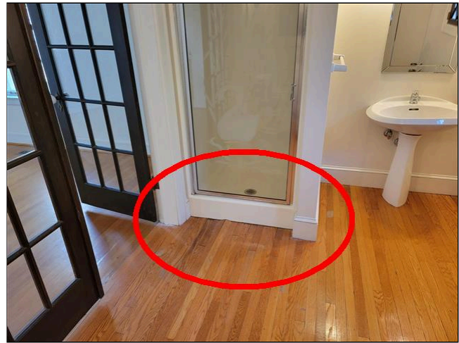
1.1 Item 2(Picture) Open Joints, Staining and Floor Disruptions (Around Primary Bathroom Shower)
