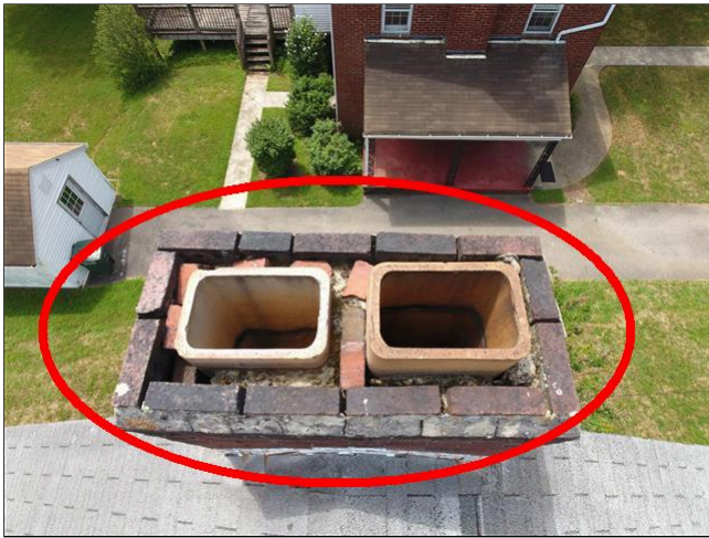
6.6 Item 1(Picture) Crown Deterioration, and Openings
