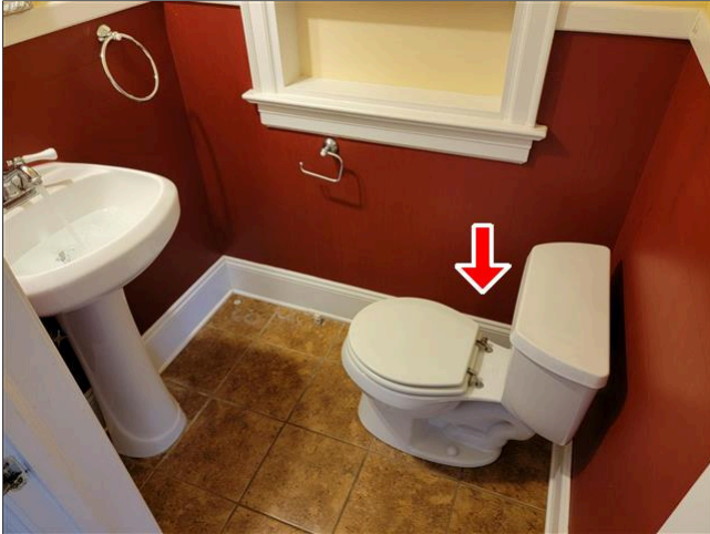
3.2 Item 1(Picture) Loose Toilet (Main Level Half Bath)
