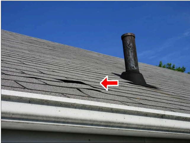
8.0 Item 5(Picture) Nail Pops (Rear)
