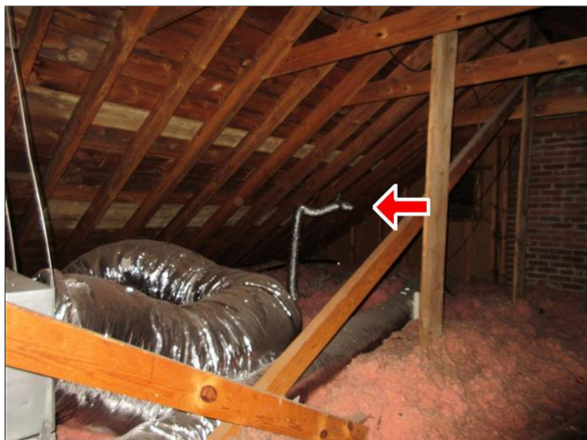
7.4 Item 1(Picture) Upstairs Bathroom Vent Discharge
