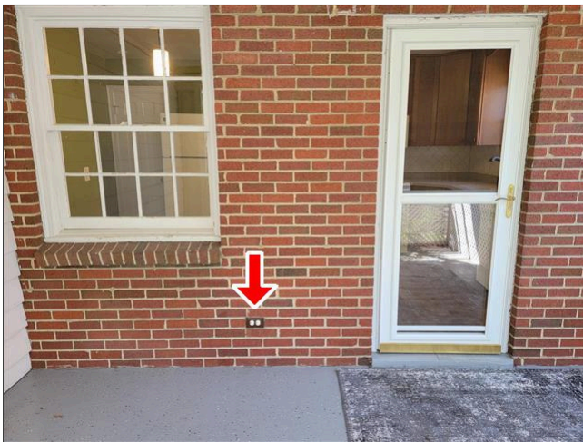
4.4 Item 7(Picture) Ungrounded Wet Location 3 Prong (Screened in Patio)
