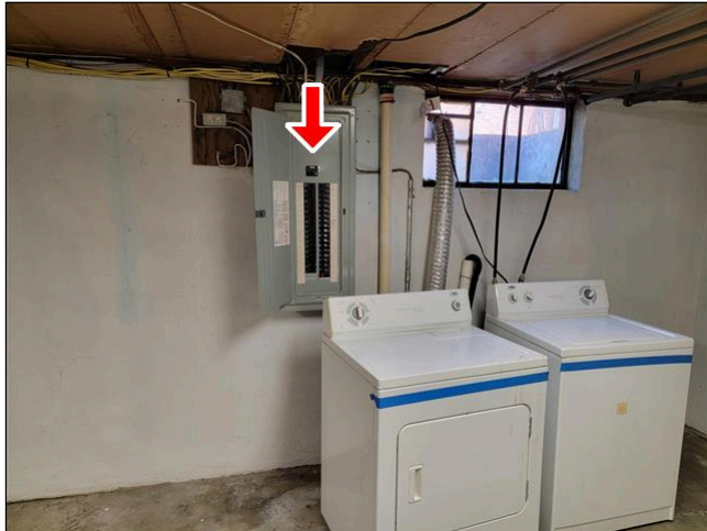
4.10 Item 1(Picture) Main Breaker
