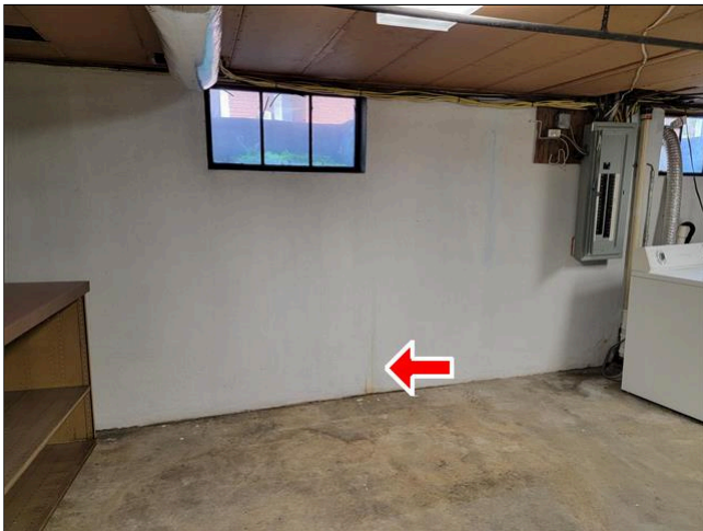
6.0 Item 1(Picture) Staining and Crack (Left Wall)
