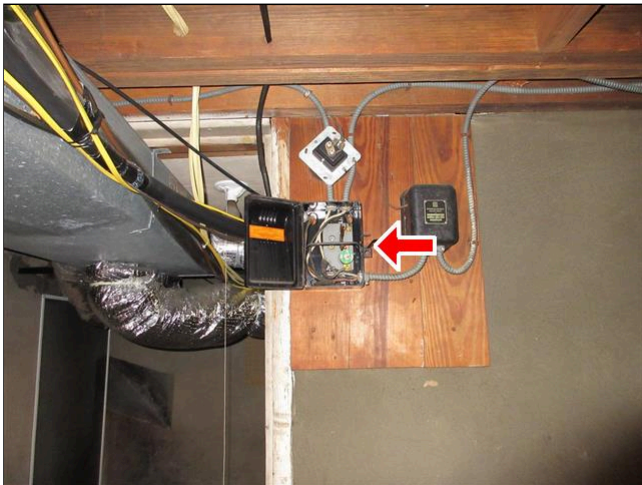
4.3 Item 1(Picture) 12 gauge wire on 30 amp fuse
