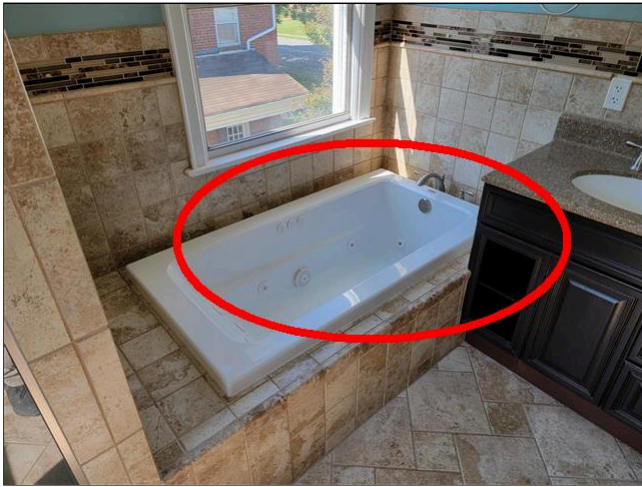
1.1 Item 1(Picture) Open Joints (Around Jet Tub)
