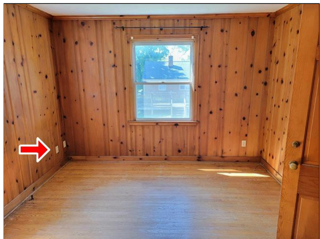
4.4 Item 4(Picture) Inactive Outlet (Main Level Right Rear Bedroom)
