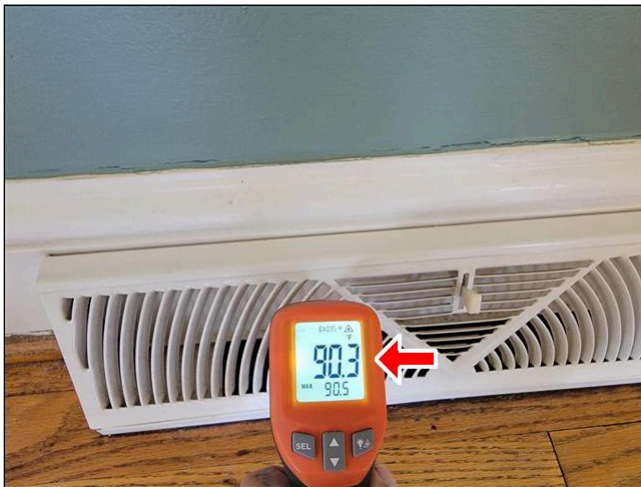
2.1.B Item 1(Picture) 90.3 Degrees (Heat Stage 1)
