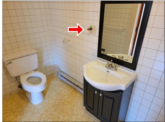
4.4 Item 6(Picture) Ungrounded Wet Location 3 Prong (Main Level Rear Bathroom)
