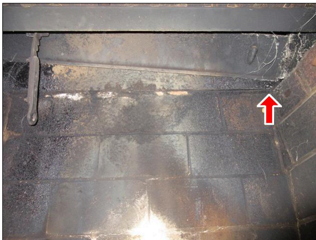
2.5.B Item 1(Picture) View of Damper
