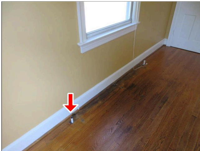
2.0.B Item 1(Picture) Uncapped Radiator Line (Multiple Locations)
