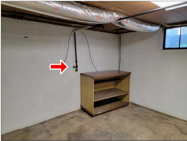
3.6 Item 1(Picture) Main Valve
