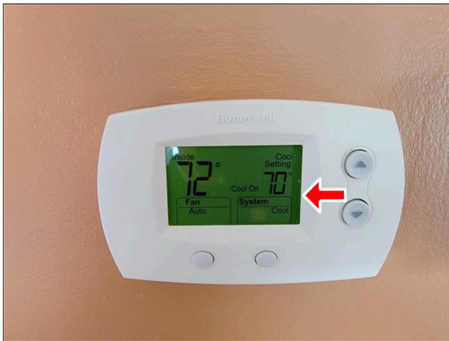
2.10.B Item 3(Picture) Thermostat Setting
