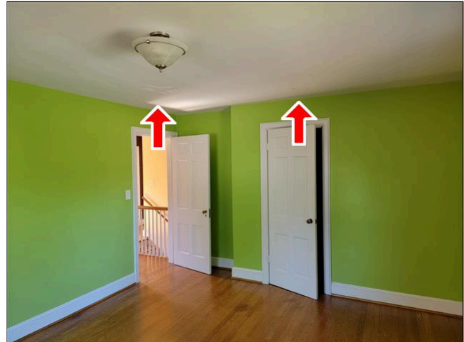
1.0 Item 2(Picture) Wet Staining (Upstairs Front Left Bedroom)
