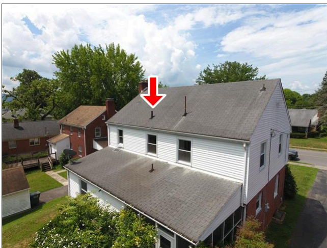
8.2 Item 1(Picture) Failed Seal
