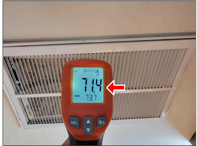
2.10.A Item 2(Picture) 71.4 Degrees (Return Temperature)
