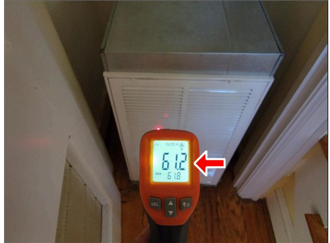
2.10.B Item 2(Picture) 61.3 Degrees (Return Temperature)
