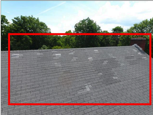
8.0 Item 1(Picture) Wind Lift, Exposed Nail Heads, and Openings (Front View)
