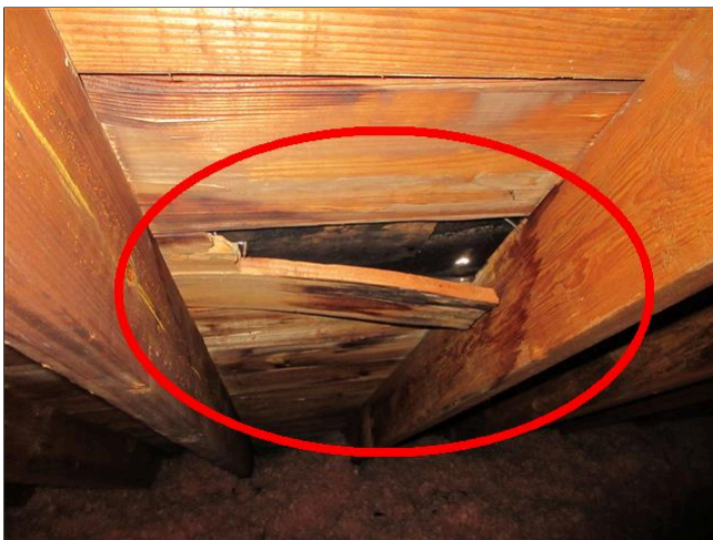
8.0 Item 3(Picture) Hole and Staining (Multiple Attic Locations)
