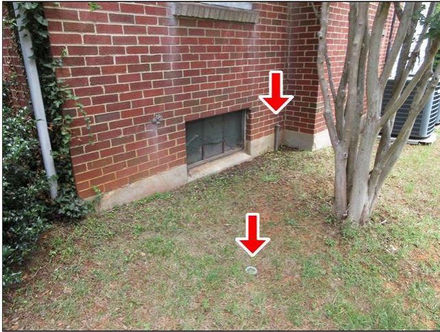
3.4 Item 1(Picture) Fill Neck and Vent (Right Side)
