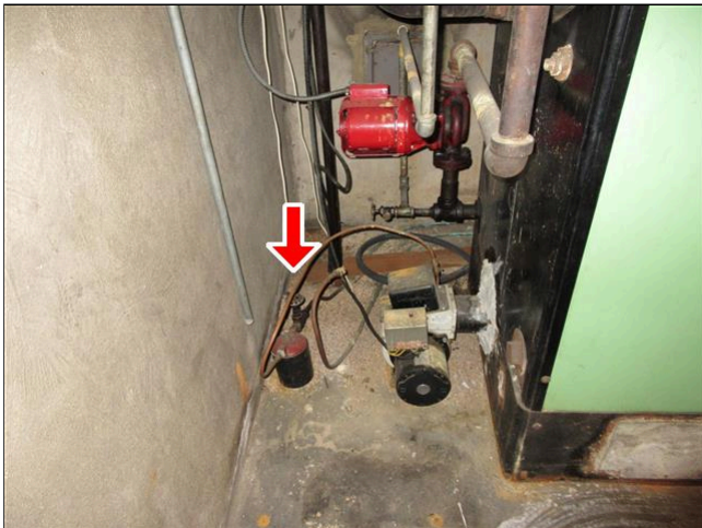
3.7 Item 1(Picture) Main Valve
