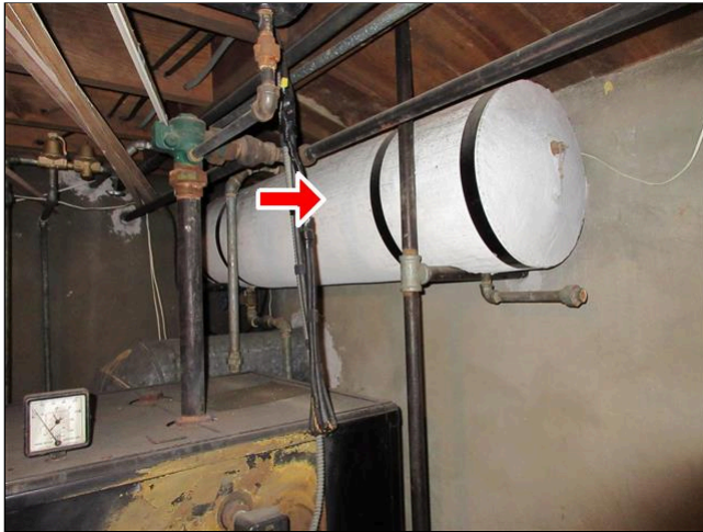
2.0.B Item 3(Picture) Potential Asbestos Material
