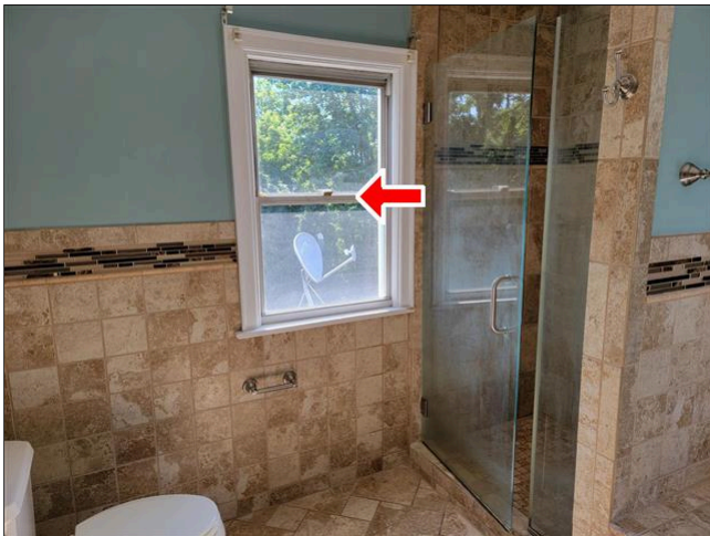
1.6 Item 3(Picture) Missing Hardware (Upstairs Bathroom)
