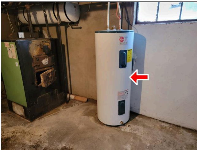
3.5 Item 1(Picture) Water Heater
