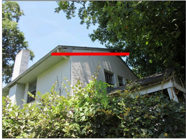
9.0 Item 2(Picture) Bare Wood and Peeling Paint (Rear Rake Board)
