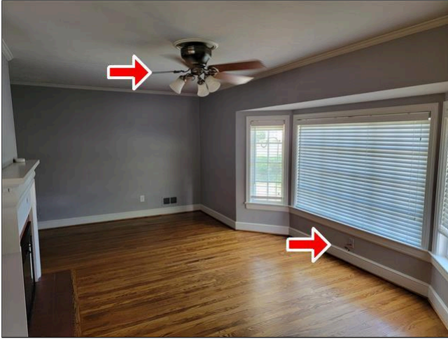
4.4 Item 5(Picture) Same Circuit (Living Room Ceiling Fan and Outlet)
