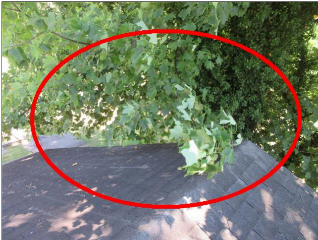
9.4 Item 1(Picture) Overgrowth (Rear)
