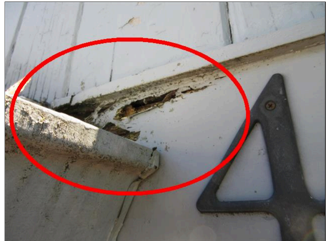
8.1 Item 4(Picture) View of the Deterioration
