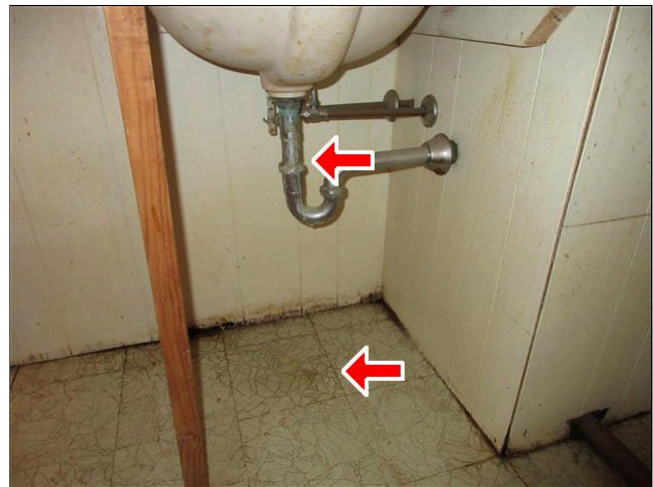
3.2 Item 8(Picture) Additional View of Leak (Below Basement Bathroom Sink)
