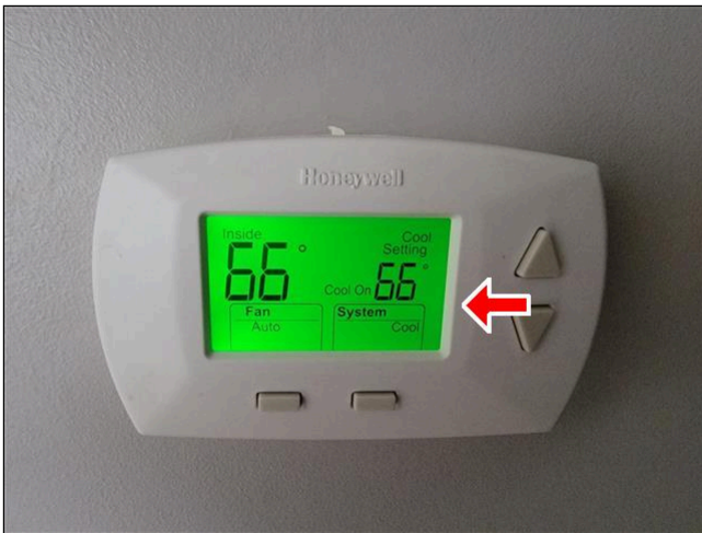
2.10 Item 3(Picture) Thermostat Setting
