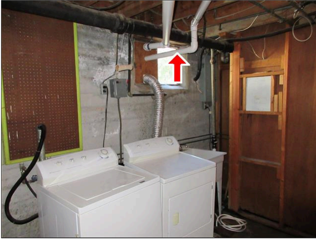
3.0 Item 3(Picture) Galvanized Corrosion (Under Kitchen)
