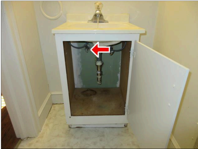
3.2 Item 5(Picture) Missing Handle (Primary Bedroom Half Bath Sink)
