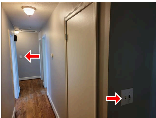
4.4 Item 1(Picture) Hall Light Switch Combination
