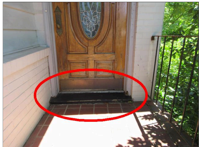
1.9 Item 2(Picture) Openings and Deterioration (Around Front Entrance)
