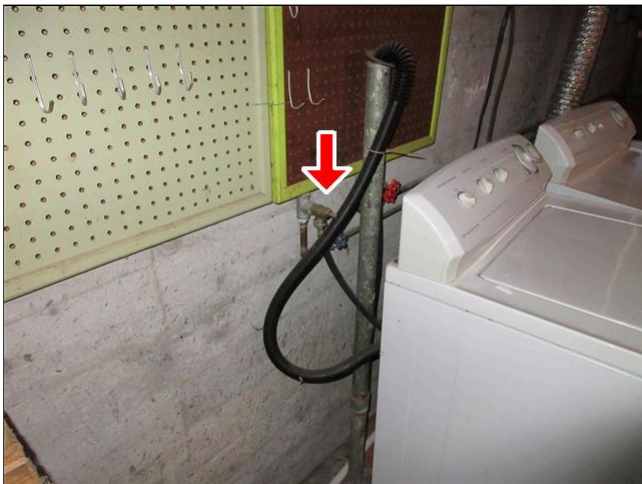
3.2 Item 9(Picture) Missing Handle (Basement Washing Machine)
