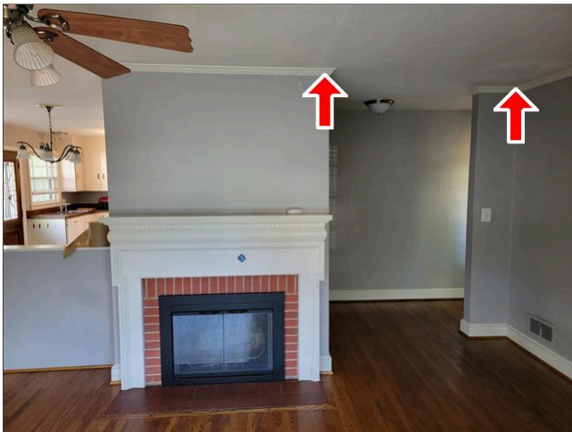
1.0 Item 3(Picture) Staining and Repairs (Living Room)
