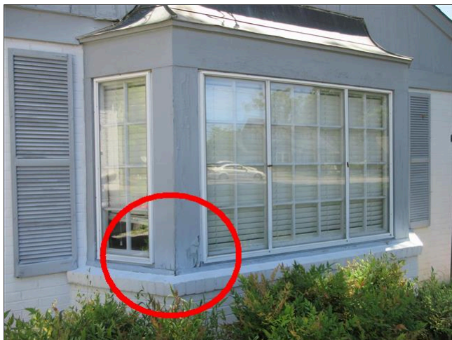
9.0 Item 5(Picture) Deterioration (Front)
