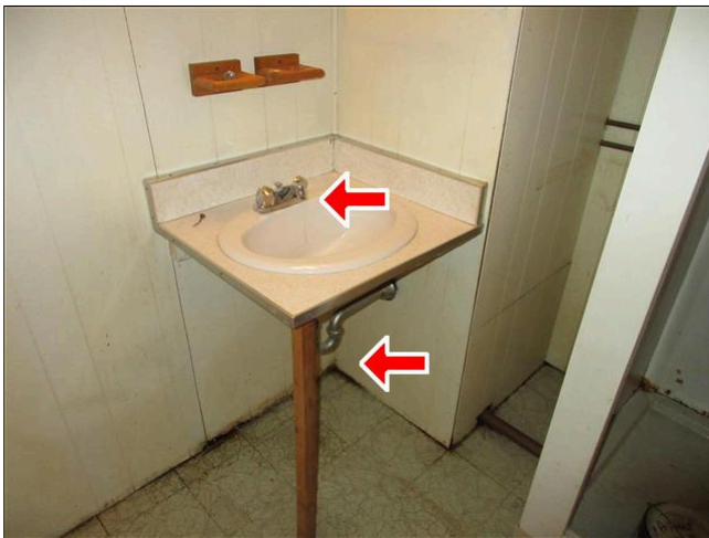
3.2 Item 7(Picture) Constant Drip and Leaking Connections (Basement Bathroom Sink)
