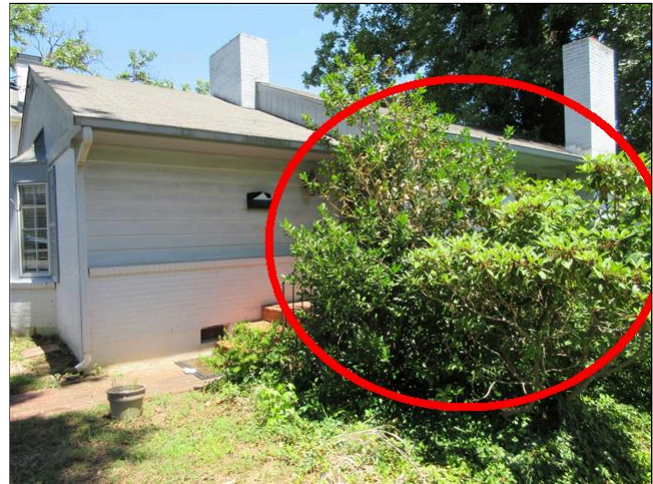
9.4 Item 2(Picture) Overgrowth (Right Side)
