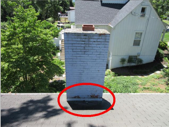
8.1 Item 1(Picture) Flashing Openings (Right Side Chimney)
