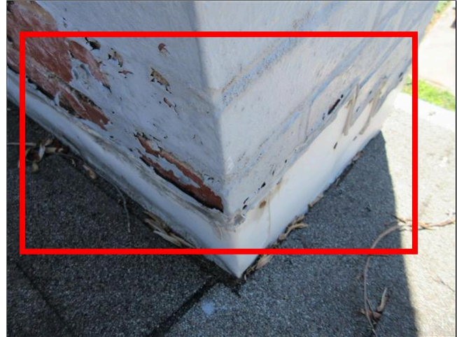
8.1 Item 2(Picture) Additional View of the Openings
