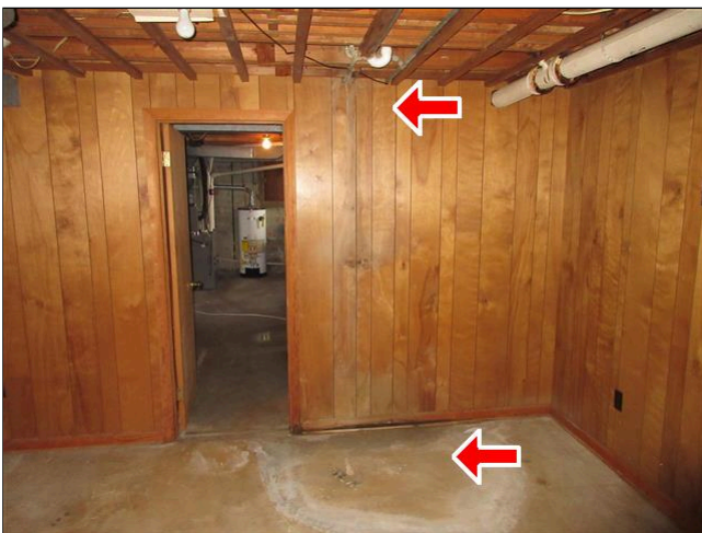
1.9 Item 7(Picture) Staining
