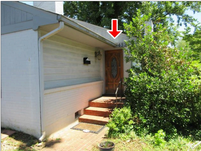
8.1 Item 3(Picture) Above Front Entrance
