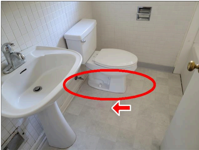
3.2 Item 1(Picture) Staining and Elevated Moisture (Main Bathroom Toilet)
