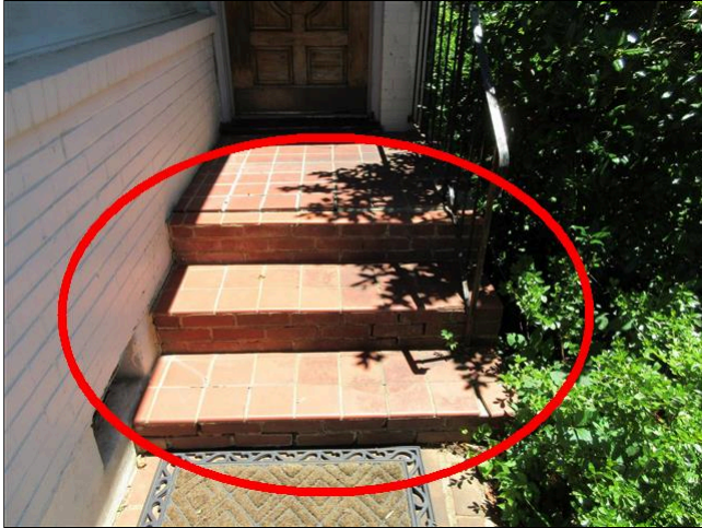
9.3 Item 1(Picture) Loose Tile (Front Stoop)
