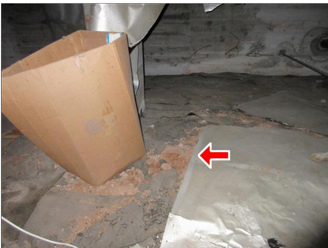
7.2 Item 1(Picture) Deterioration and Exposed Soil
