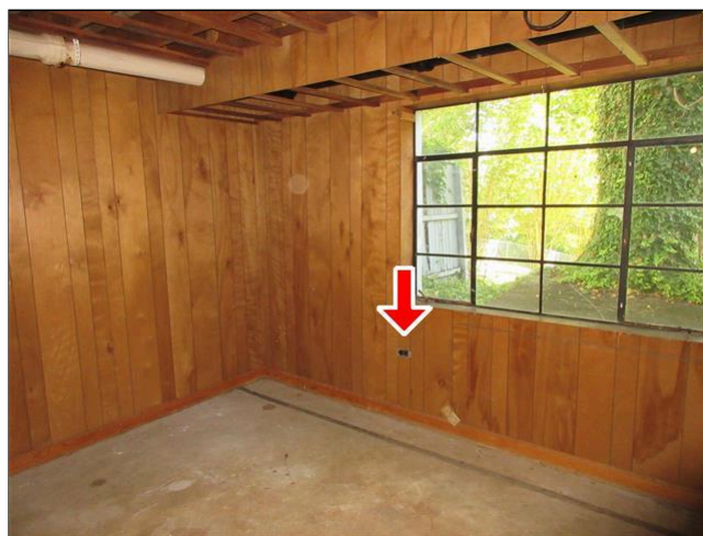
4.4 Item 4(Picture) Broken Outlet (Rear Basement Bedroom)
