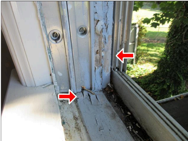
9.2 Item 1(Picture) Bare Wood and Peeling Paint (Most Windows)
