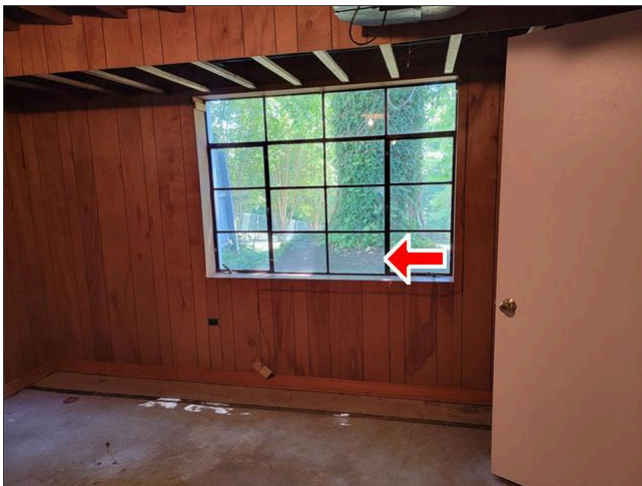
1.6 Item 1(Picture) Cracked Glass and Seized Windows (Left Rear Basement Bedroom)
