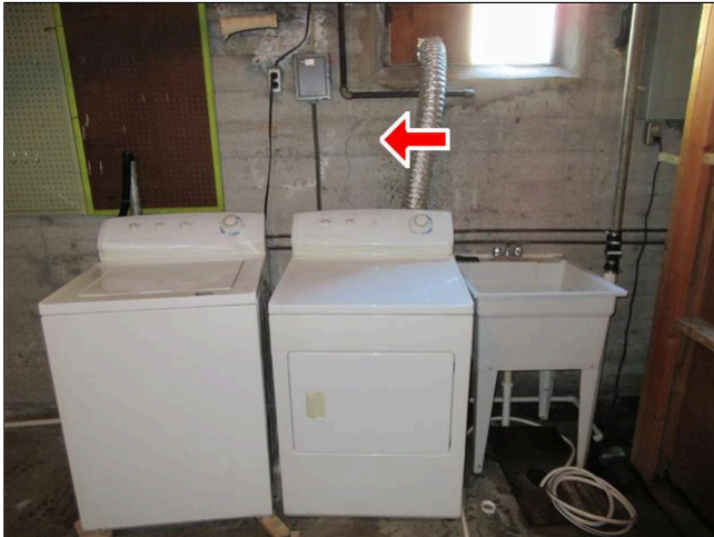
6.0 Item 1(Picture) Crack and Staining (Basement Left Wall)
