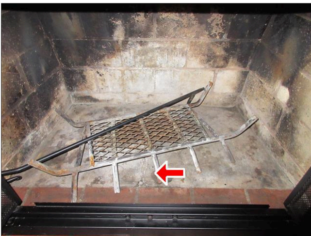
2.6 Item 1(Picture) Cracking (Living Room Fireplace)
