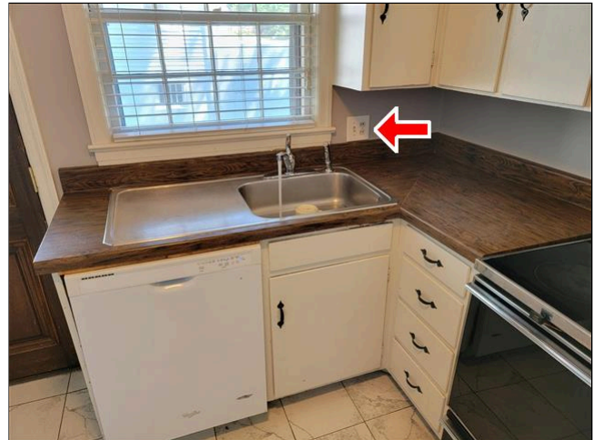
4.5 Item 2(Picture) Ungrounded 2 Prong (Kitchen)
