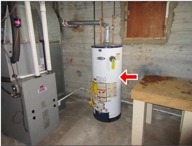
3.6 Item 1(Picture) Water Heater
