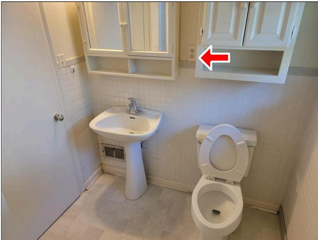
4.5 Item 1(Picture) Ungrounded 3 Prong (Main Bathroom)
