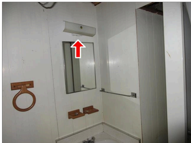
4.5 Item 3(Picture) Grounded 3 Prong (Basement Bathroom)
