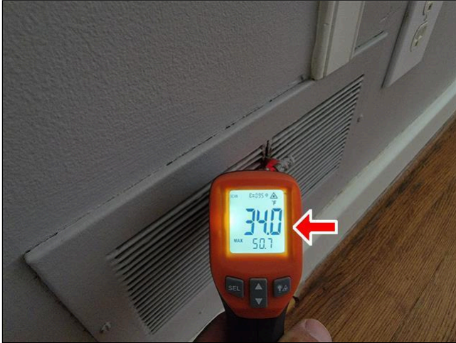
2.10 Item 1(Picture) 34 Degrees (Supply Temperature)
