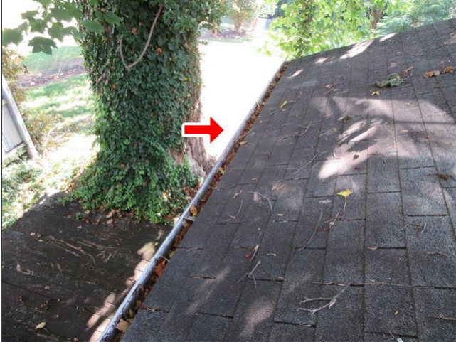
8.3 Item 1(Picture) Debris (Rear Patio Roof)
