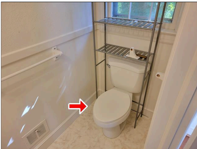
3.2 Item 3(Picture) Loose Toilet (Primary Bedroom Half Bath)
