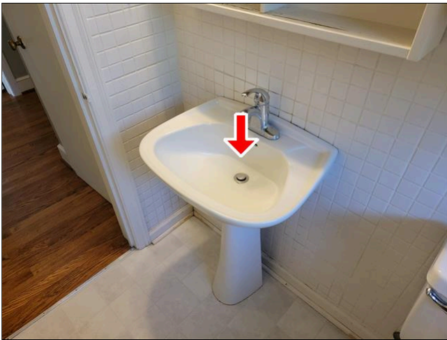
3.0 Item 5(Picture) Slow Drain (Main Bathroom Sink)
