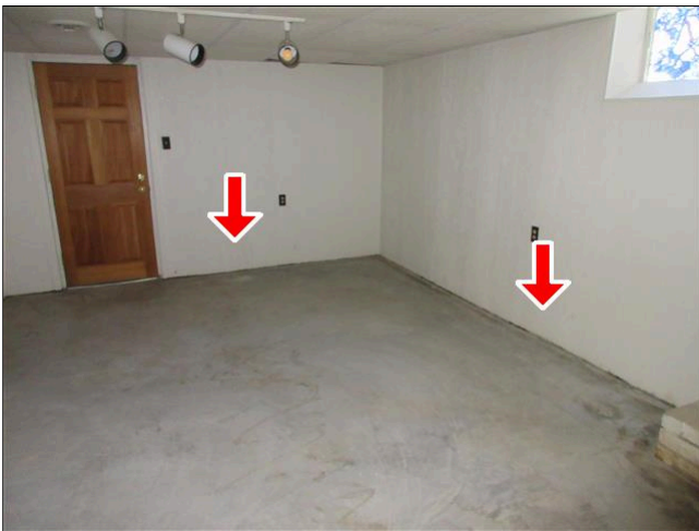
1.9 Item 5(Picture) Staining and Moisture (Basement Den)
