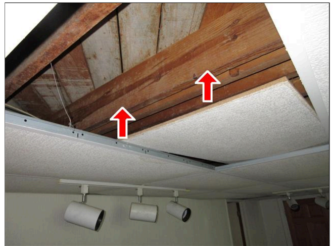
1.9 Item 6(Picture) Organic Growth (Behind Basement Ceiling Panels)
