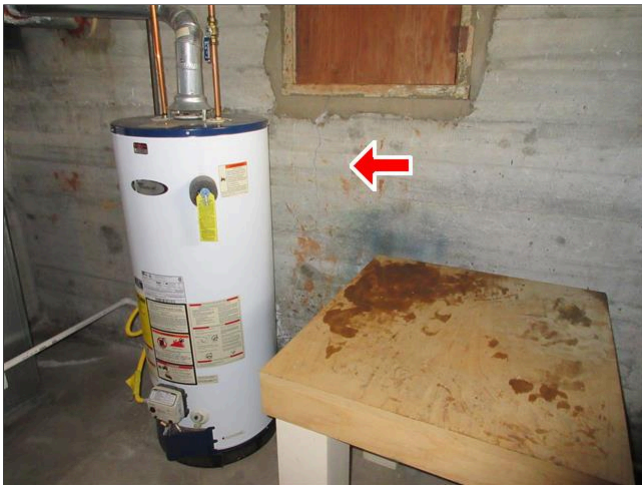
6.0 Item 3(Picture) Crack (Below Crawl Space Entrance)
