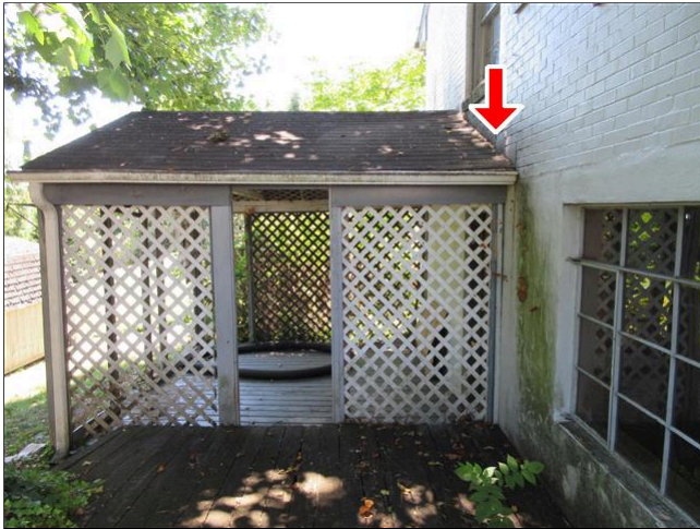
8.3 Item 3(Picture) Improperly Sloped (Rear)
