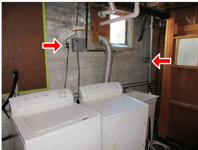
4.5 Item 4(Picture) Grounded 3 Prong (Basement Laundry Room)
