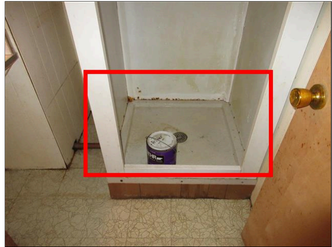
3.2 Item 6(Picture) Rust/Corrosion (Basement Bathroom Shower)
