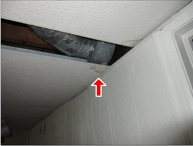
2.3 Item 3(Picture) Condensation Causing Ceiling Staining
