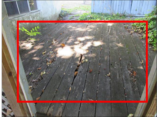
9.3 Item 2(Picture) Deteriorated Deck Boards
