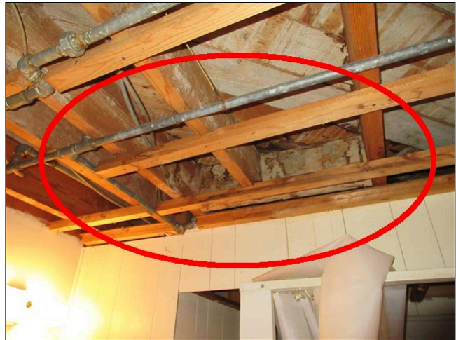
3.2 Item 2(Picture) Staining and Moisture (Below Main Bathroom Toilet)
