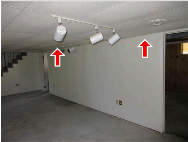
1.0 Item 5(Picture) Staining (Basement Den - Multiple Locations)
