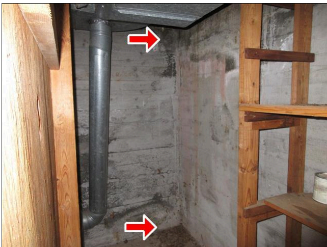
1.9 Item 1(Picture) Staining and Elevated Moisture (Below Front Entrance)
