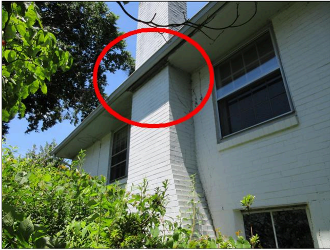
9.0 Item 1(Picture) Openings (Around Right Side Chimney)
