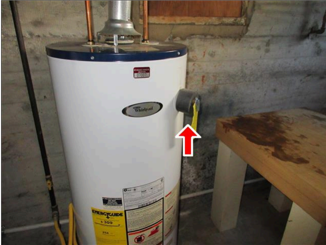
3.3 Item 1(Picture) No Discharge Tube
