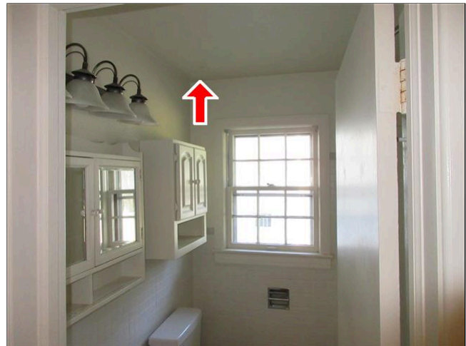
1.0 Item 4(Picture) Disruptions (Main Bathroom Ceiling)
