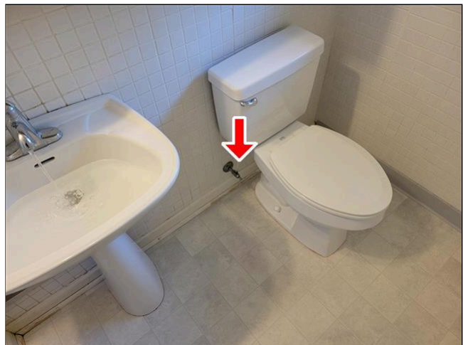
3.2 Item 4(Picture) Missing Handle (Main Bathroom Toilet)
