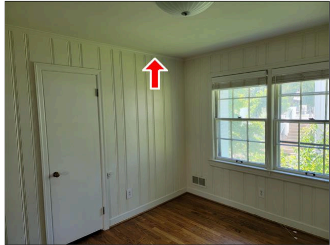
1.0 Item 2(Picture) Staining (Front Right Bedroom)
