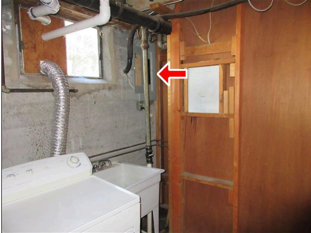
4.10 Item 1(Picture) Main Electrical Distribution Panel
