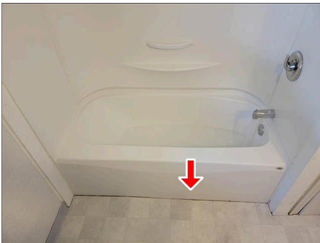
1.2 Item 1(Picture) Open Joint (Around Main Bathroom Tub)
