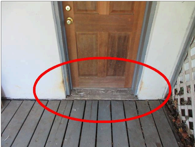
9.0 Item 3(Picture) Deterioration and Openings (Around Basement Entrance)
