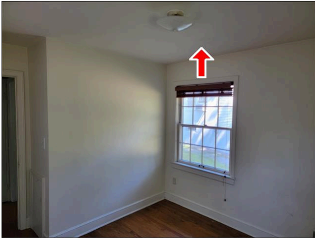
1.0 Item 1(Picture) Staining (Left Rear Bedroom)
