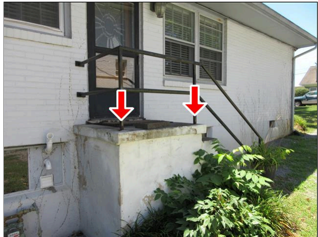
9.3 Item 4(Picture) Deteriorated Posts and Baluster Spacing (Left Side)
