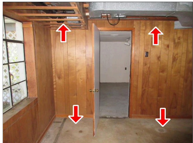
3.0 Item 2(Picture) Staining and Drips (Multiple Locations)
