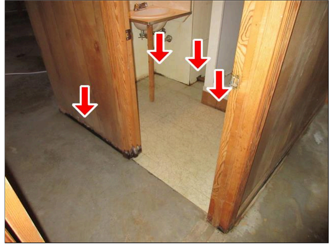
1.9 Item 4(Picture) Staining (Multiple Locations Around the Basement Bathroom)
