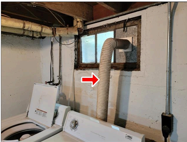
7.3 Item 1(Picture) Vinyl Ducting
