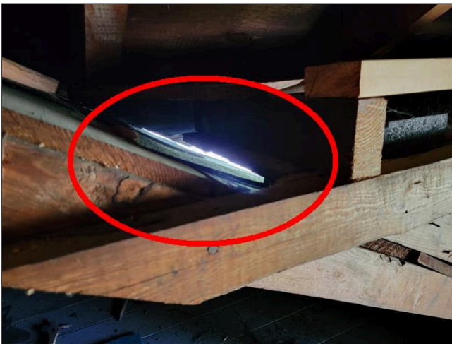
1.7 Item 1(Picture) Gaps/Daylight (Multiple Locations)
