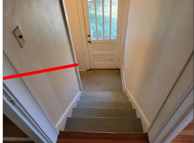
1.3 Item 2(Picture) No Graspable Handrail (Basement Stairwell - Multiple Locations)
