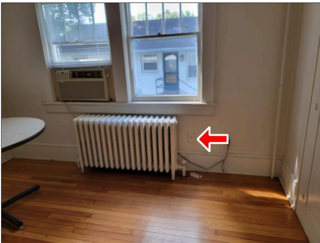
4.4 Item 1(Picture) Inactive 220 Outlet (Dining Room)
