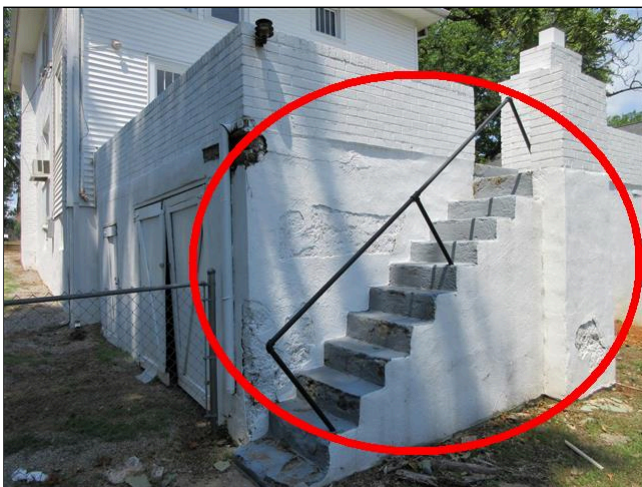
9.3 Item 1(Picture) No Balusters (Rear)
