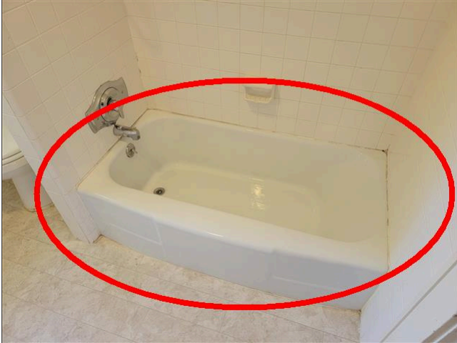
1.1 Item 6(Picture) Open Joints (Around Upstairs Bathroom Tub)
