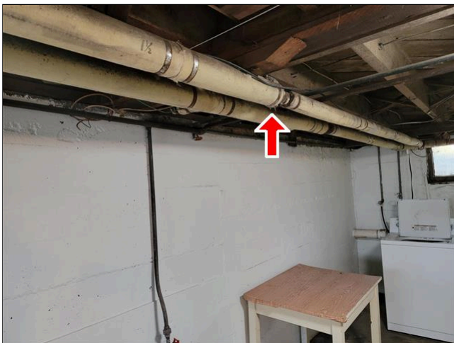
2.2 Item 1(Picture) Potential Asbestos Pipe Insulation
