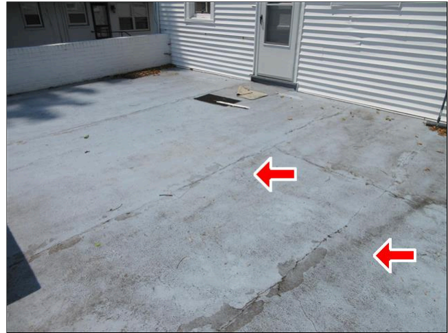
6.0 Item 6(Picture) Cracking Patio Slab (Multiple Locations)
