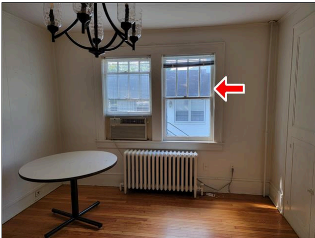
1.6 Item 7(Picture) Cracked Glass (Dining Room)
