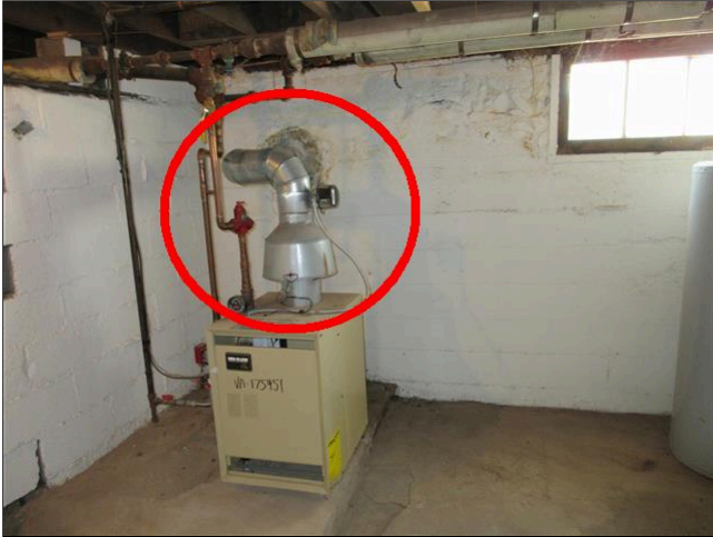
1.1 Item 3(Picture) Wall Staining and Elevated Moisture (Behind Boiler)
