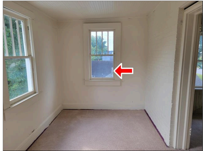
1.6 Item 4(Picture) Cracked Glass (Upstairs Right Rear Bedroom)
