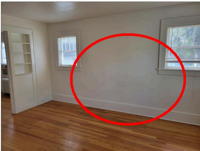
1.1 Item 1(Picture) Staining and Elevated Moisture (Living Room)
