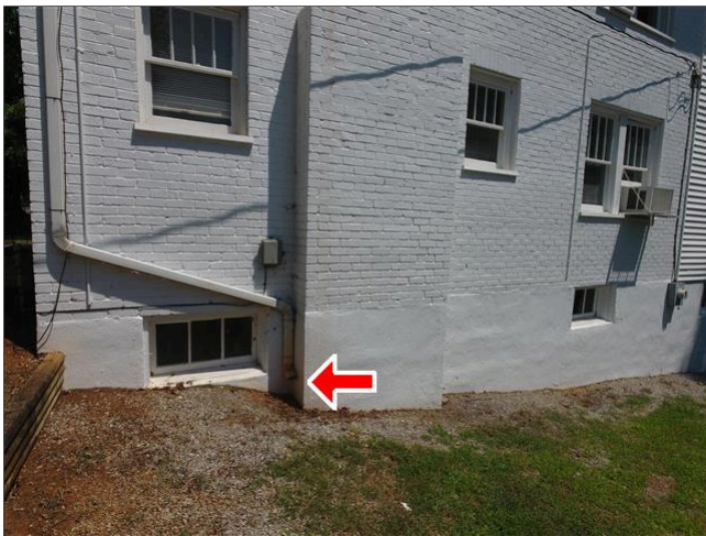
8.3 Item 1(Picture) Discharge (Right Side)
