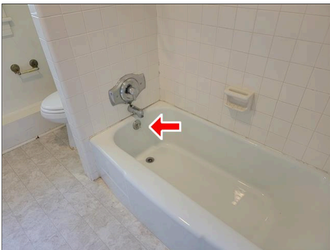
3.2 Item 1(Picture) Not Sealing (Upstairs Bathroom)
