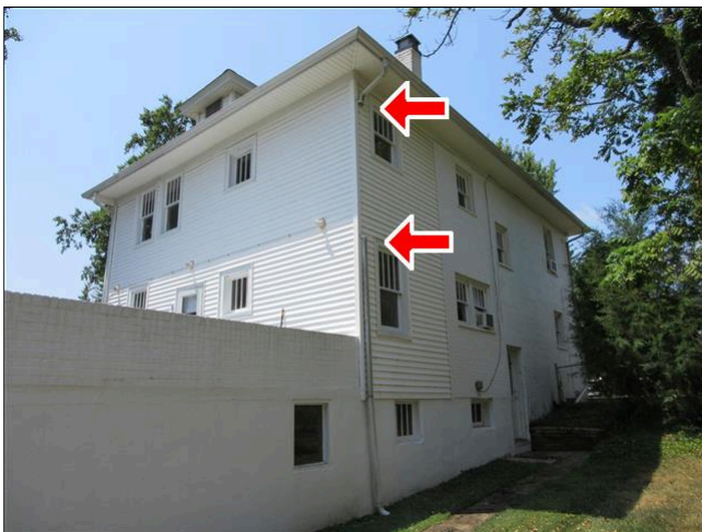
8.3 Item 3(Picture) Missing Downspout (Left Rear)
