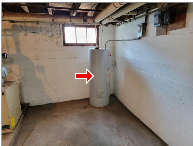
3.5 Item 1(Picture) Water Heater
