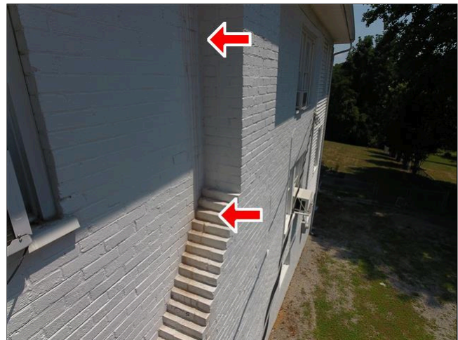
1.1 Item 2(Picture) Staining (Exterior View)
