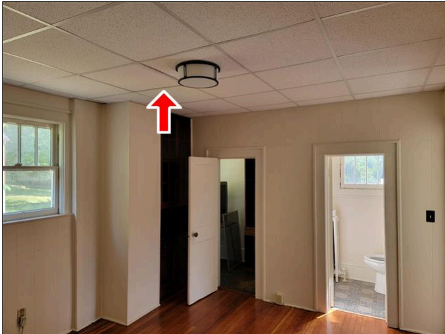
1.0 Item 1(Picture) Staining (Den - Bathroom Above)
