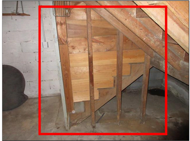
1.9 Item 5(Picture) Insect Damage (Under Steps - Multiple Locations)
