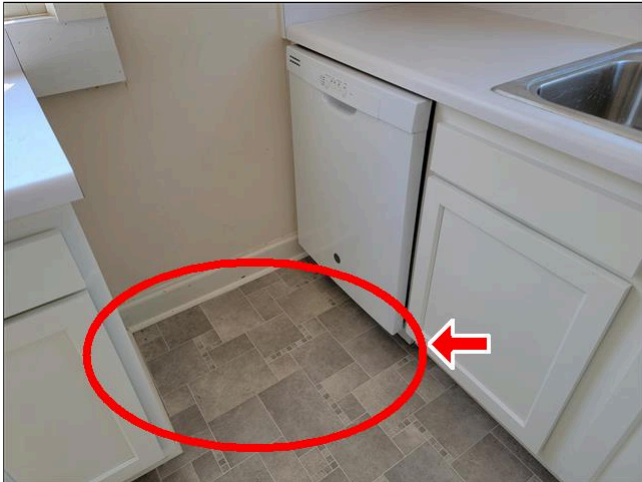
5.0 Item 1(Picture) Leak/Water
