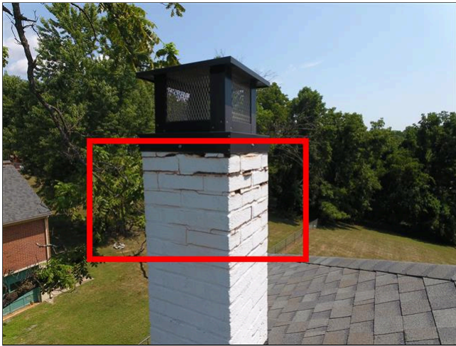
6.6 Item 1(Picture) Mortar Joint Deterioration (Left Chimney)
