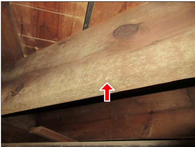
1.9 Item 3(Picture) Organic Growth (Multiple Floor Joists)
