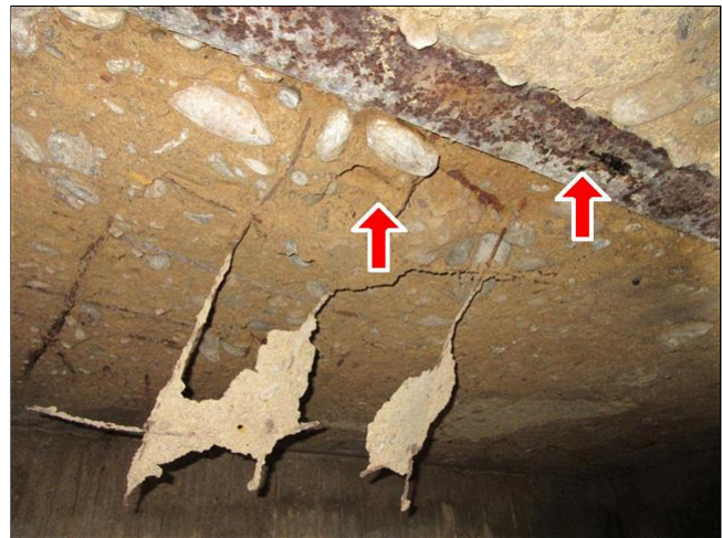
6.0 Item 8(Picture) Deterioration and Exposed Metal (Multiple Locations)
