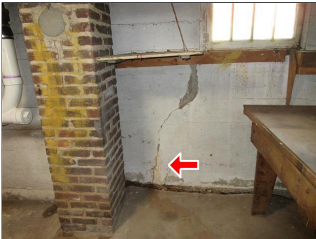
6.0 Item 3(Picture) Crack and Staining (Left Wall)
