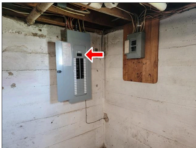
4.10 Item 1(Picture) Main Breaker
