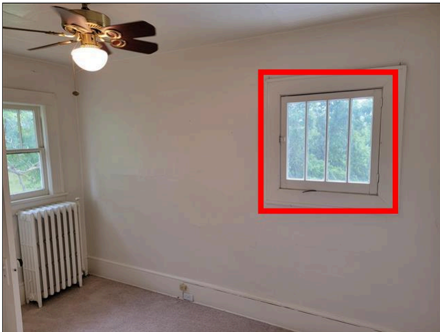
1.6 Item 1(Picture) Gaps/Air Leaks (Multiple Locations)
