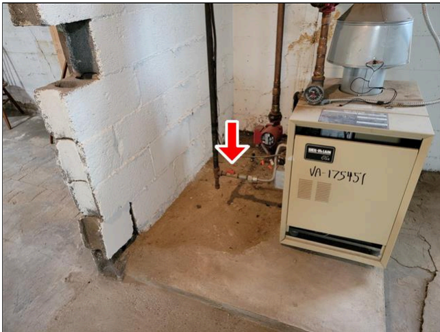
3.8 Item 1(Picture) Gas Boiler Valve
