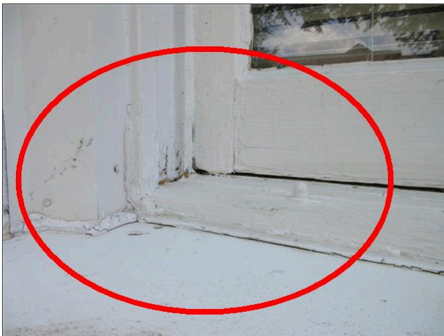
9.0 Item 3(Picture) Open Joints and Gaps (Around Windows)
