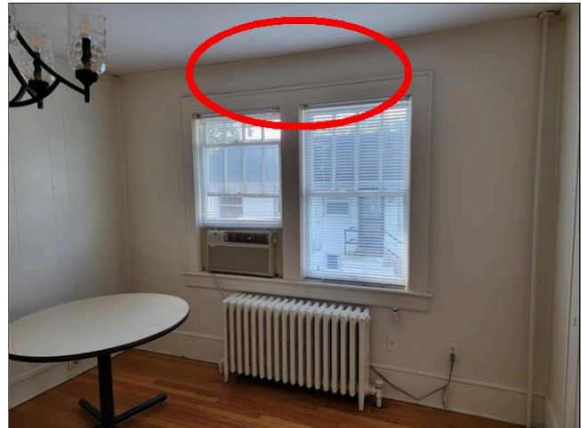
1.1 Item 5(Picture) Staining (Dining Room - Staining Upstairs)
