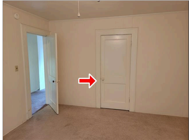
1.5 Item 2(Picture) Not Latching/Painted Latch (Upstairs Front Right Bedroom Closet)
