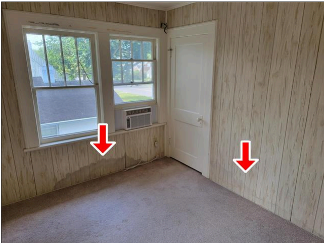
1.1 Item 4(Picture) Staining (Upstairs Right Side Bedroom)
