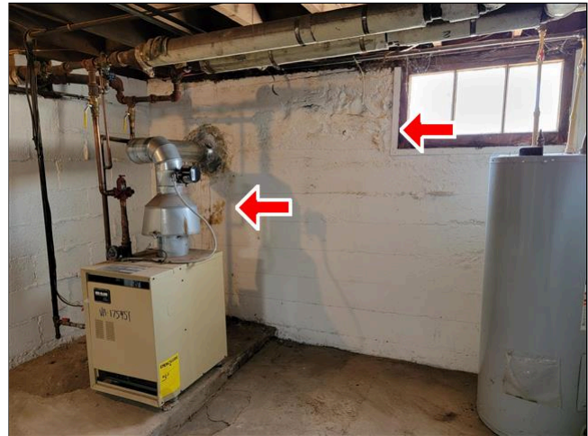
1.9 Item 2(Picture) Staining and Elevated Moisture
