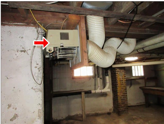
4.4 Item 5(Picture) Active but Non-Functional Ventilation Fan (Basement)
