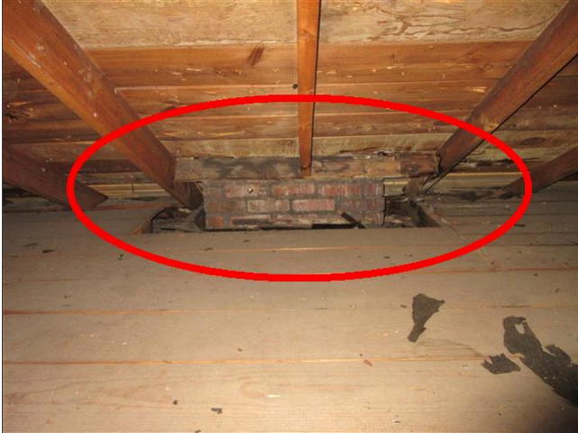
1.7 Item 2(Picture) Staining and Recent Repairs (Around Right Chimney)
