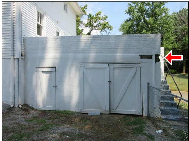
9.0 Item 4(Picture) Deterioration From Gutter (Right Rear)
