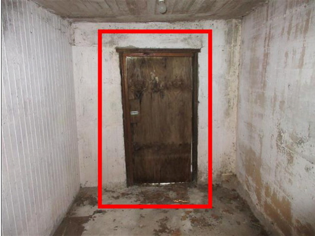
9.1 Item 1(Picture) Gaps and Daylight (Basement)
