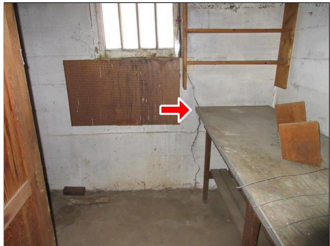
6.0 Item 4(Picture) Crack and Displacement (Right Wall)
