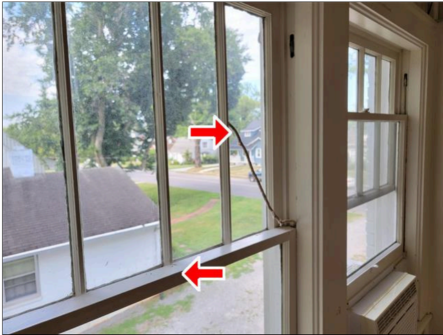
1.6 Item 3(Picture) Missing Lock and Broken Balance Cord (Multiple Locations)
