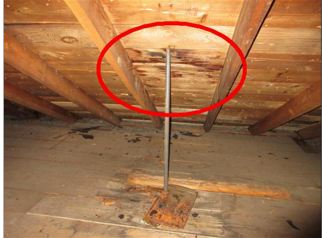
1.7 Item 3(Picture) Staining (Around Vent Pipes)
