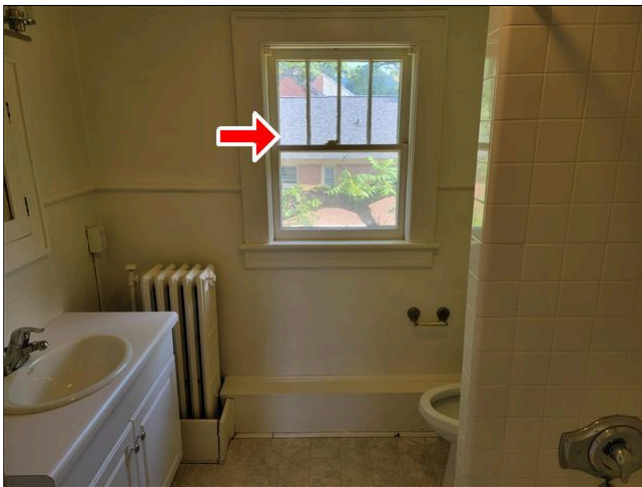
1.6 Item 5(Picture) Cracked Glass (Upstairs Bathroom)
