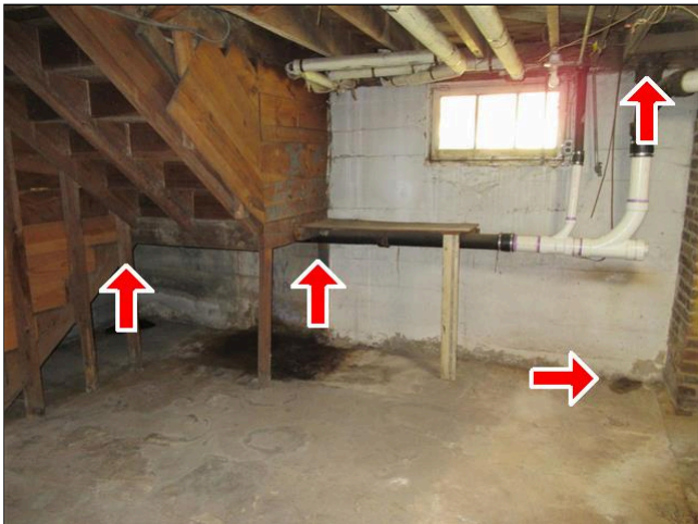
3.0 Item 3(Picture) Cracked and Leaking
