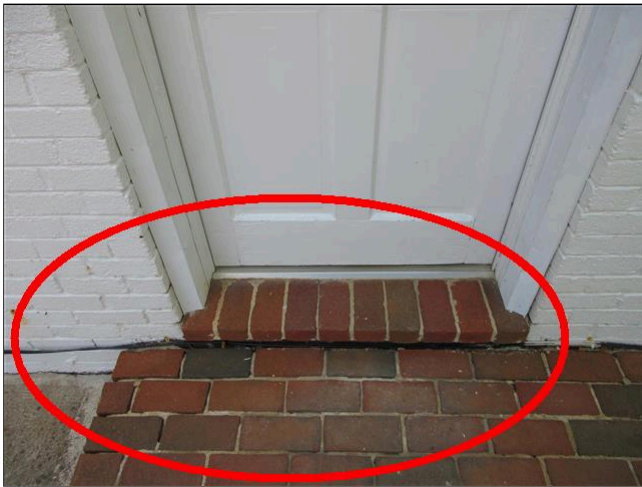
9.0 Item 1(Picture) Open Joints (Around Entrances and Stoop)
