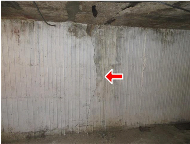
6.0 Item 5(Picture) Crack (Rear Storage Room)
