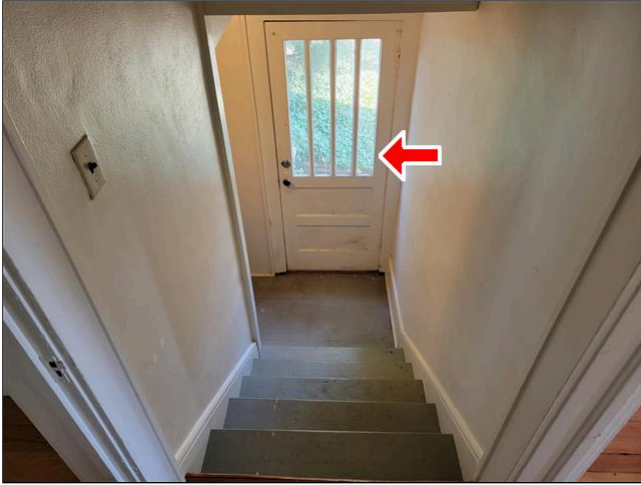
1.6 Item 9(Picture) No Safety Glass (Stairwell Landing)
