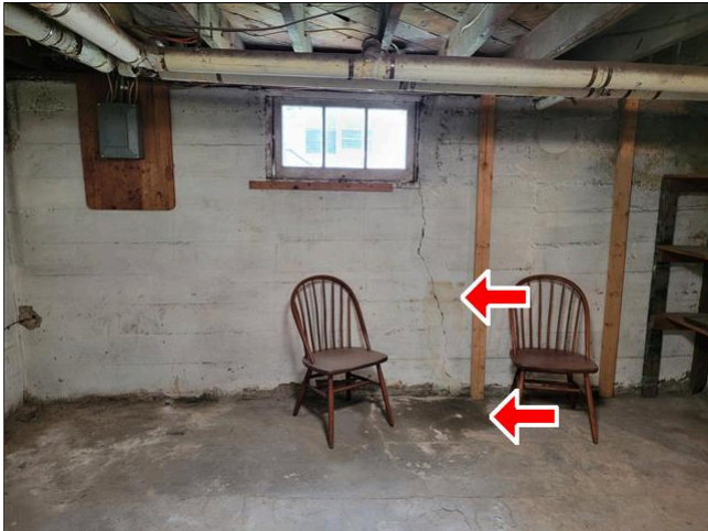
6.0 Item 1(Picture) Crack and Staining (Right Wall)
