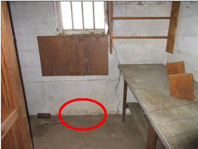
1.9 Item 8(Picture) Shelter Tubes
