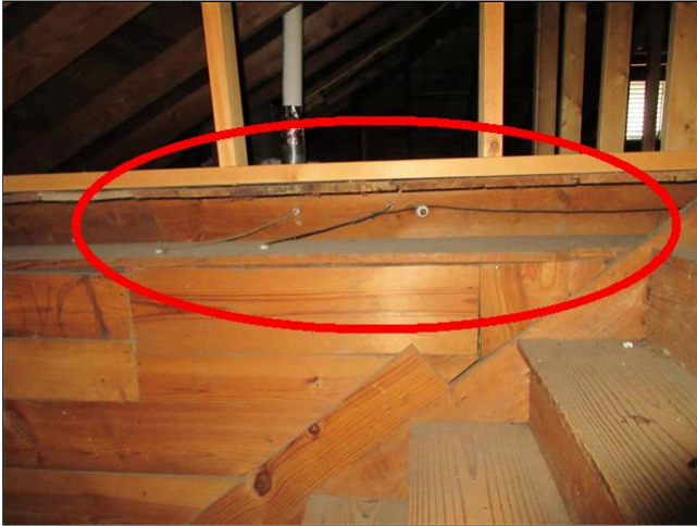
4.3 Item 1(Picture) Active Knob and Tube Wiring (Attic View)
