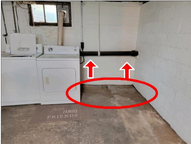
3.0 Item 1(Picture) Cracked and Leaking
