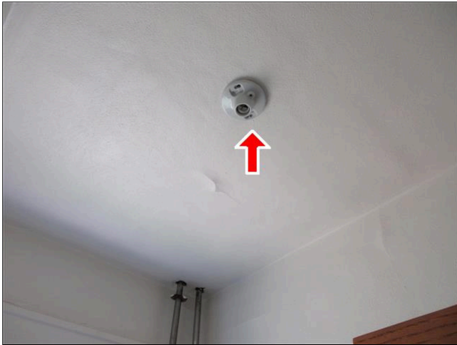
4.4 Item 3(Picture) Missing Pull Chain View
