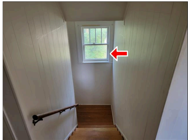
1.6 Item 6(Picture) No Safety Glass (Stairwell Landing)
