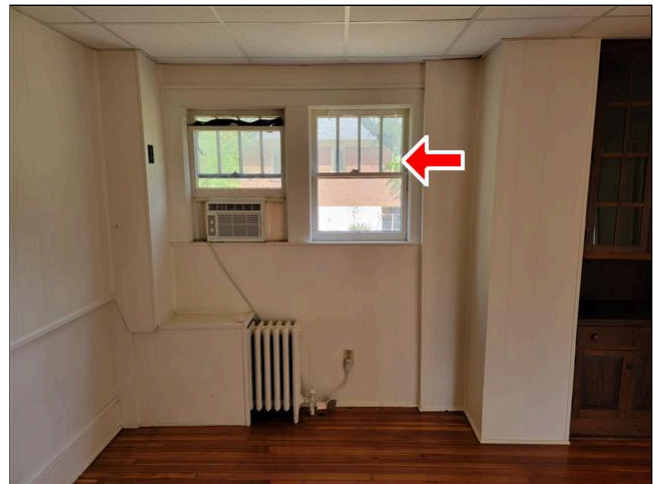
1.6 Item 8(Picture) Cracked Glass (Den)
