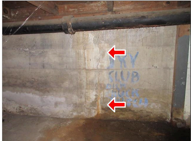
6.0 Item 2(Picture) Crack and Staining (Left Wall)
