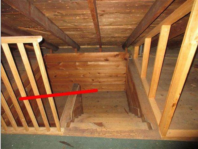
1.3 Item 1(Picture) No Graspable Handrail (Attic Stairwell - Multiple Locations)
