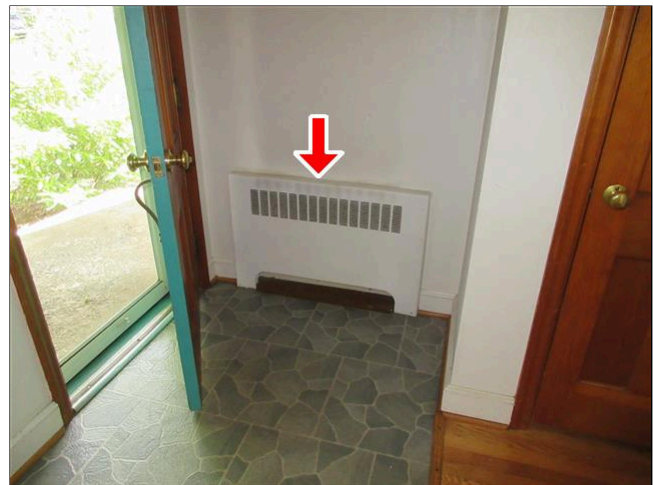
2.0 Item 4(Picture) Front Entrance (Not Functional)
