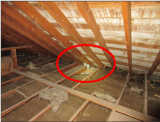
6.4 Item 1(Picture) Cut Ceiling Joist
