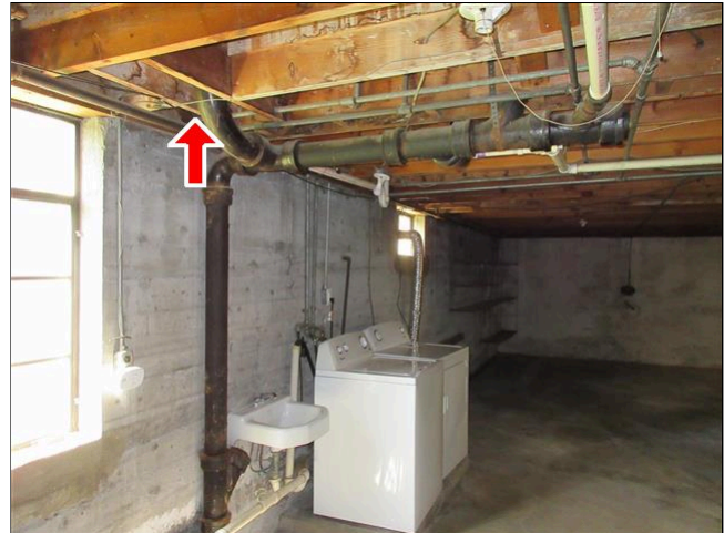
3.2 Item 2(Picture) Staining (Below Toilet)
