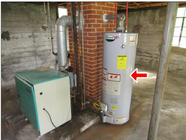
3.5 Item 1(Picture) Water Heater
