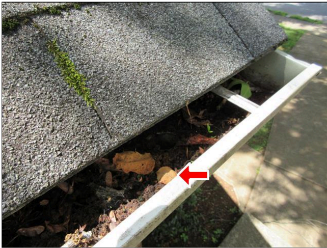
8.3 Item 1(Picture) Debris (Multiple Areas)
