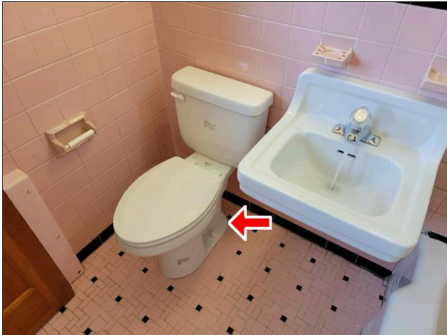
3.2 Item 1(Picture) Loose Toilet (Primary Bathroom)
