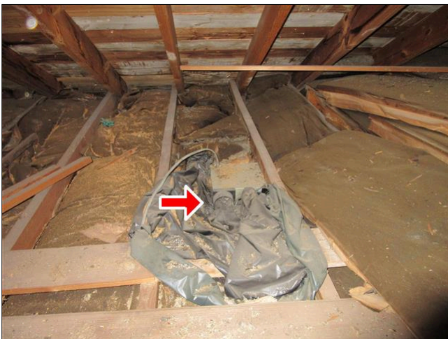
7.3 Item 1(Picture) Main Bathroom Exhaust Fan Discharge
