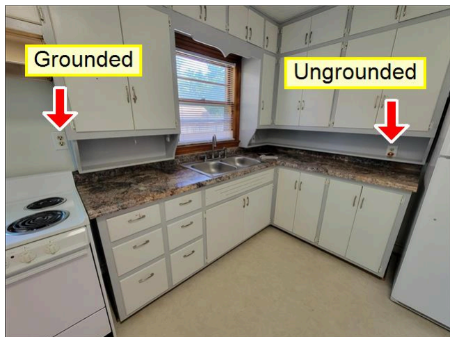
4.5 Item 1(Picture) Kitchen Outlets (Grounded & Ungrounded)
