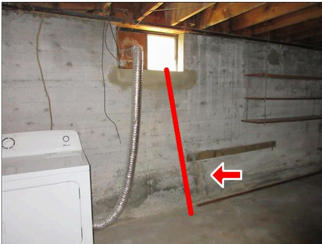
6.0 Item 1(Picture) Crack and Staining (Right Wall)
