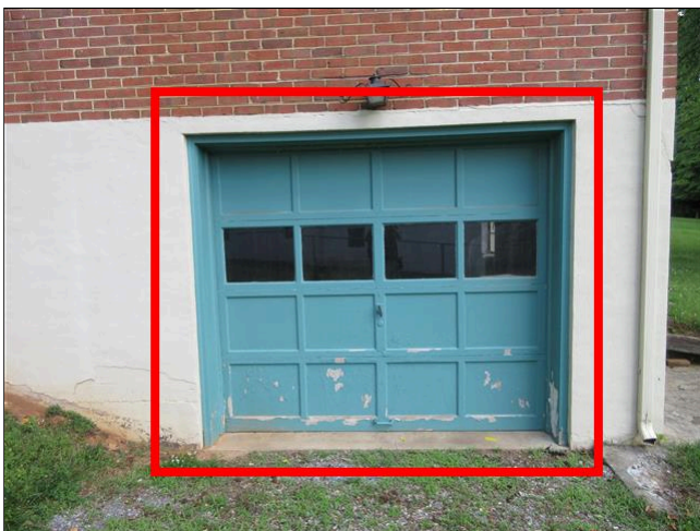
9.1 Item 3(Picture) No Weather Stripping
