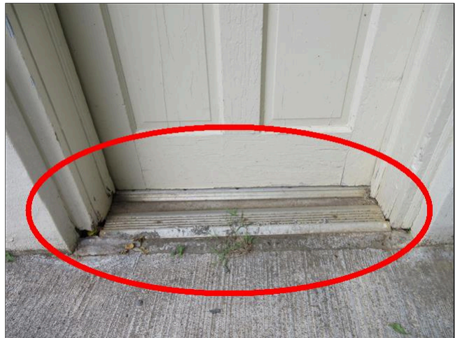
9.1 Item 2(Picture) Openings and Deterioration (Exterior View)
