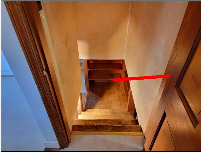
1.3 Item 1(Picture) No Handrail (Basement Stairwell)
