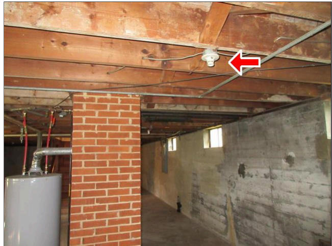
4.4 Item 4(Picture) Missing Pull Chain (Basement Light Fixture)
