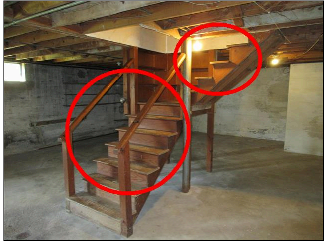
1.3 Item 2(Picture) No Balusters (Basement Stairwell)
