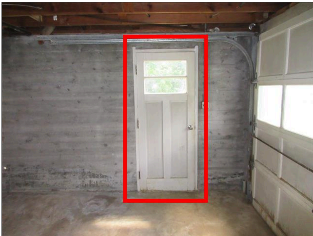
9.1 Item 1(Picture) No Weather Stripping (Interior View)
