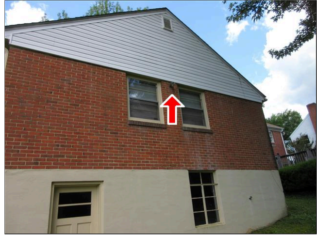
4.4 Item 6(Picture) Not Functional/Potential Failed Light Bulbs (Rear)
