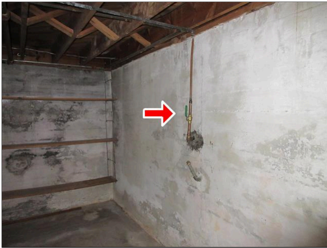
3.6 Item 1(Picture) Main Valve
