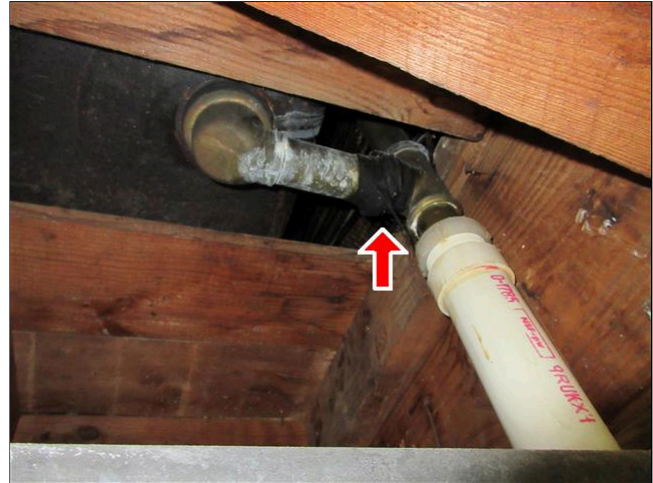
3.2 Item 9(Picture) Wrapped in Tape
