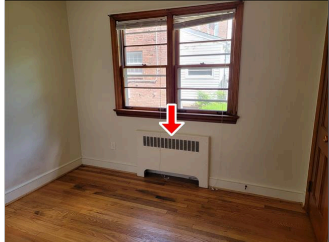
2.0 Item 2(Picture) Left Bedroom (Not Functional)
