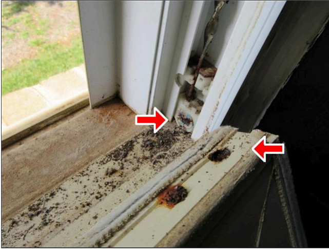
1.6 Item 4(Picture) Broken Pivot Shoe and Balance (Both Sides)
