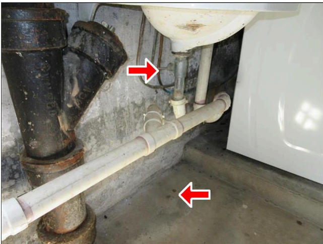
3.2 Item 6(Picture) Minor Drip (Under Basement Sink)
