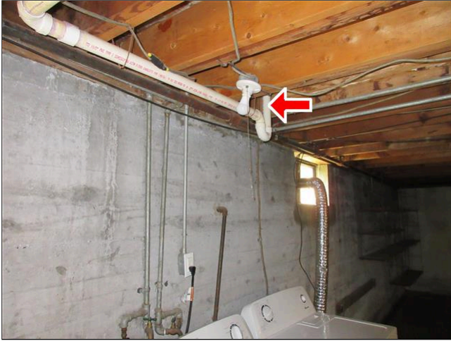
4.4 Item 5(Picture) Seized Pull Chain (Basement Light Fixture)
