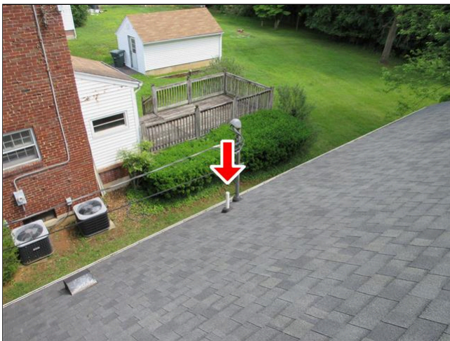
8.2 Item 1(Picture) Vent Pipe
