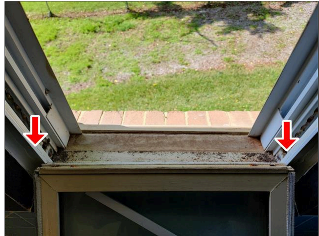
1.6 Item 3(Picture) Broken Pivot Shoe Arms (Main Bathroom)
