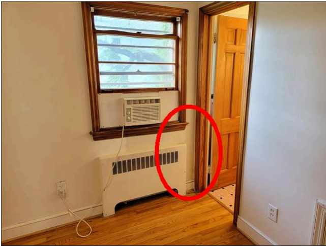
1.1 Item 1(Picture) Staining (Primary Bedroom)
