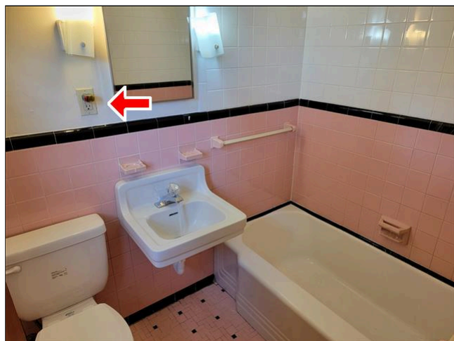
4.6 Item 1(Picture) Inactive GFCI (Primary Bathroom)
