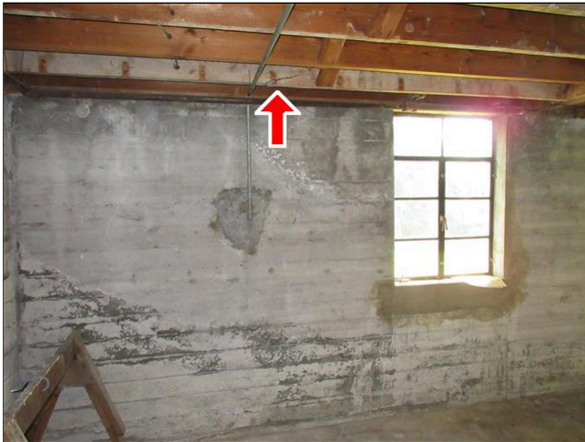
6.2 Item 1(Picture) Cracked Joist (Rear)
