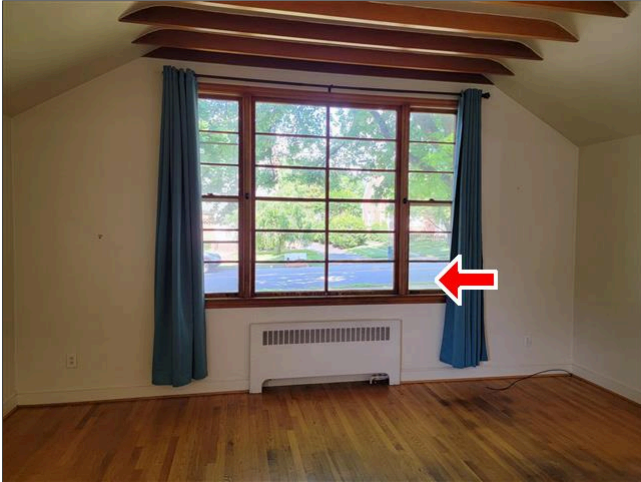
1.6 Item 1(Picture) Cracked Storm Window (Living Room)
