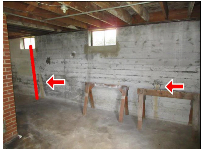
6.0 Item 2(Picture) Crack and Staining (Left Wall)
