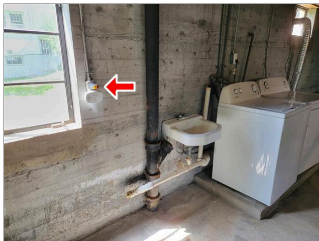
4.5 Item 2(Picture) Basement Sink Outlet (Grounded)
