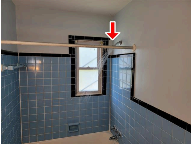
3.2 Item 10(Picture) Dripping Shower Head (Main Bathroom)
