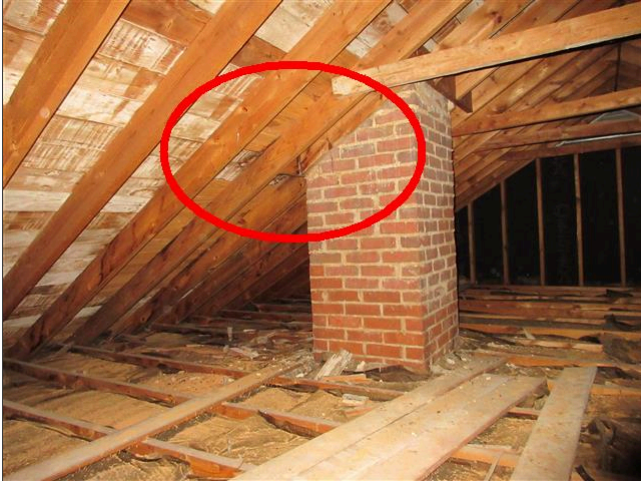
1.7 Item 1(Picture) Staining and Repairs (Around Chimney)
