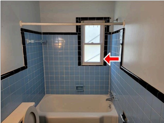
1.6 Item 2(Picture) No Safety Glass and Broken Pivot Shoe Arms (Main Bathroom)
