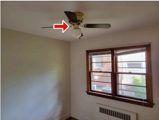
4.4 Item 3(Picture) Missing Light Pull Chain (Left Side Bedroom)
