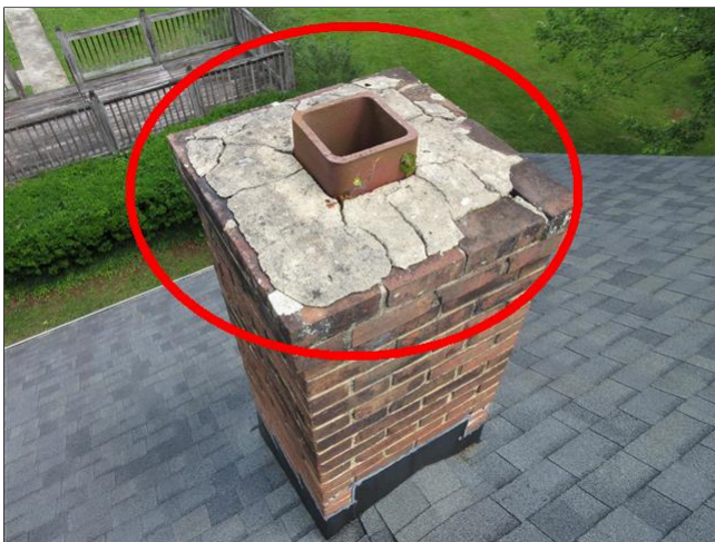
6.6 Item 1(Picture) Cracked/Worn Crown and Openings
