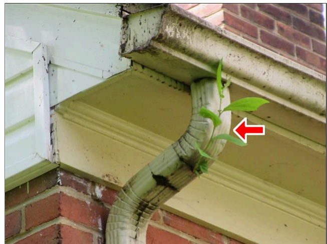
8.3 Item 4(Picture) Additional View of Overgrowth
