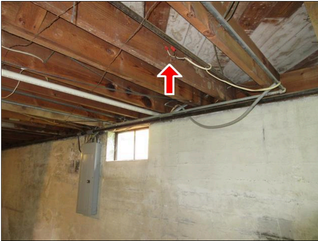
4.4 Item 7(Picture) No Junction Box (Basement)
